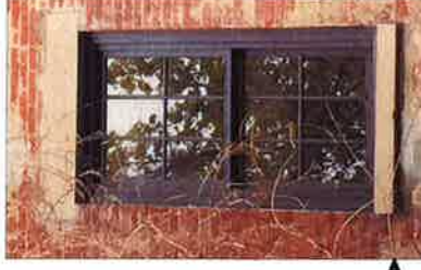
REMOVE Painted 6-Over-6 Wood Double Hung Windows - No Change In Existing Masonry Opening
