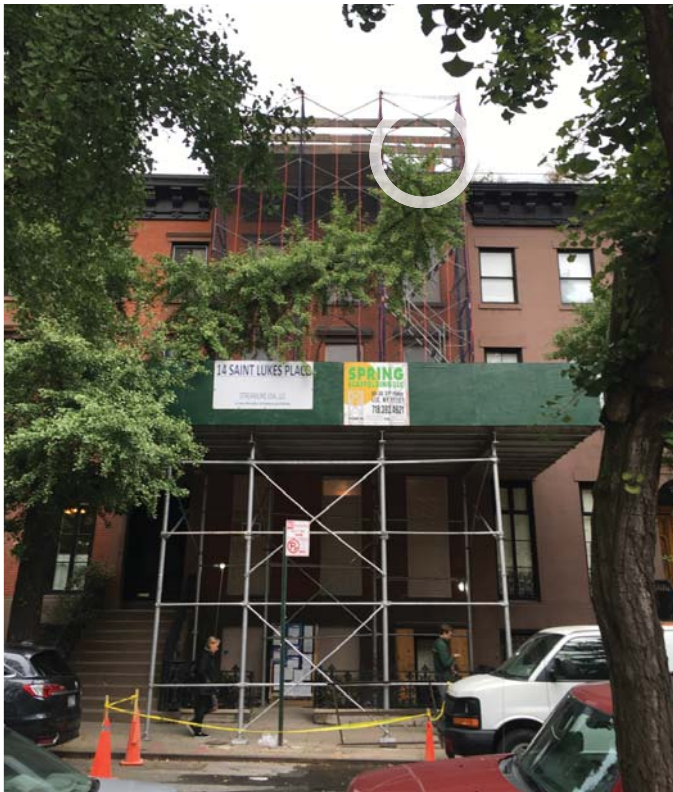
VIEW 1 ROOFTOP ADDITION NOT EXPECTED TO BE VISIBLE FLUE: SOME VISIBILITY EXPECTED
