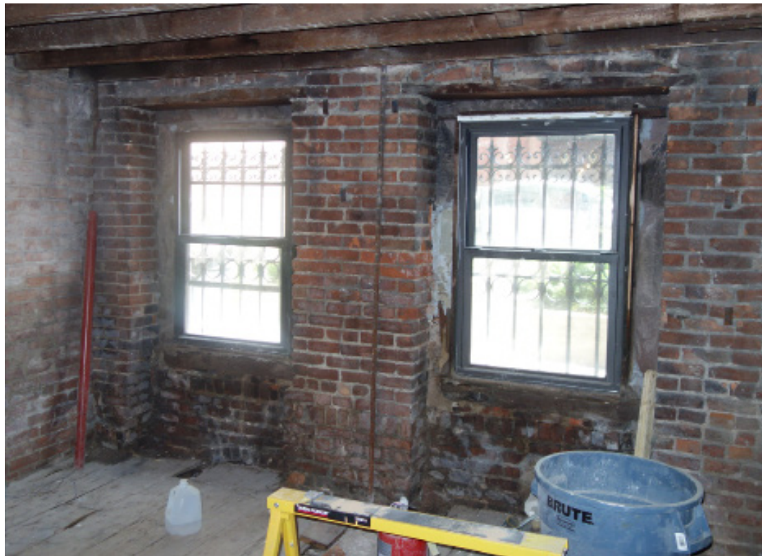
EXISTING DETERIORATED BRICK South (Front) Facade
