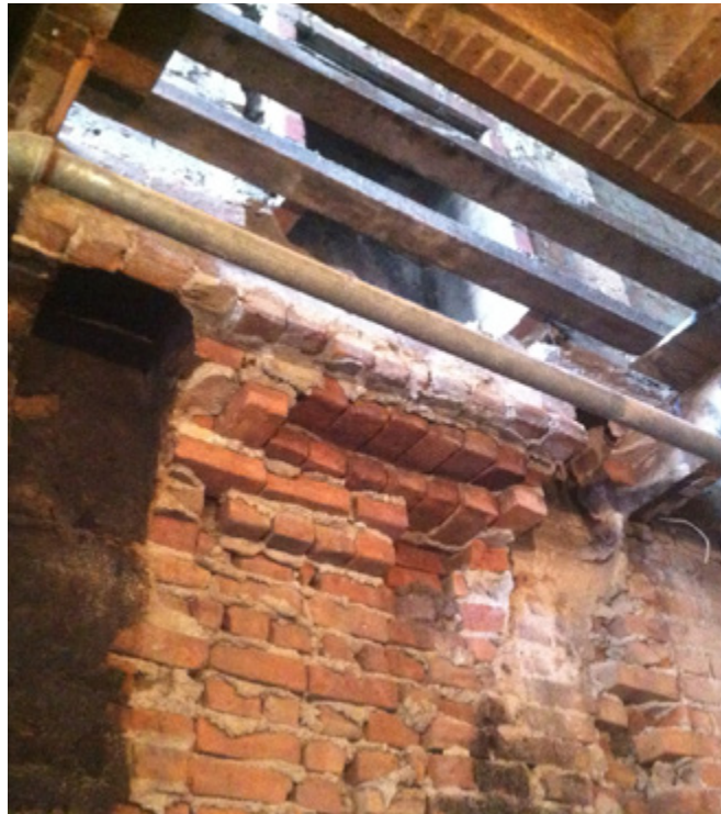
EXISTING DETERIORATED BRICK East Wall
