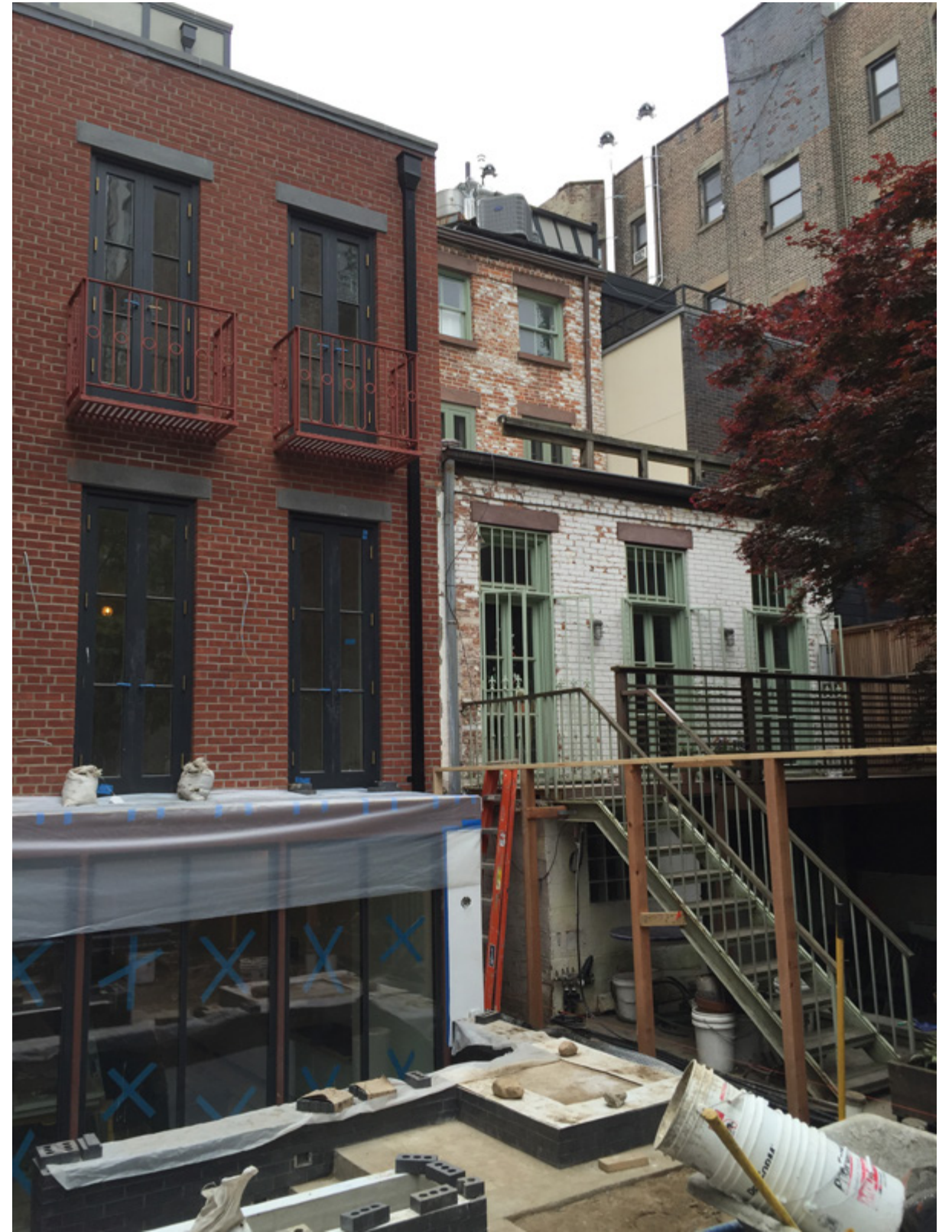
REAR FACADE Basement through Second Floor and Adjoining property
