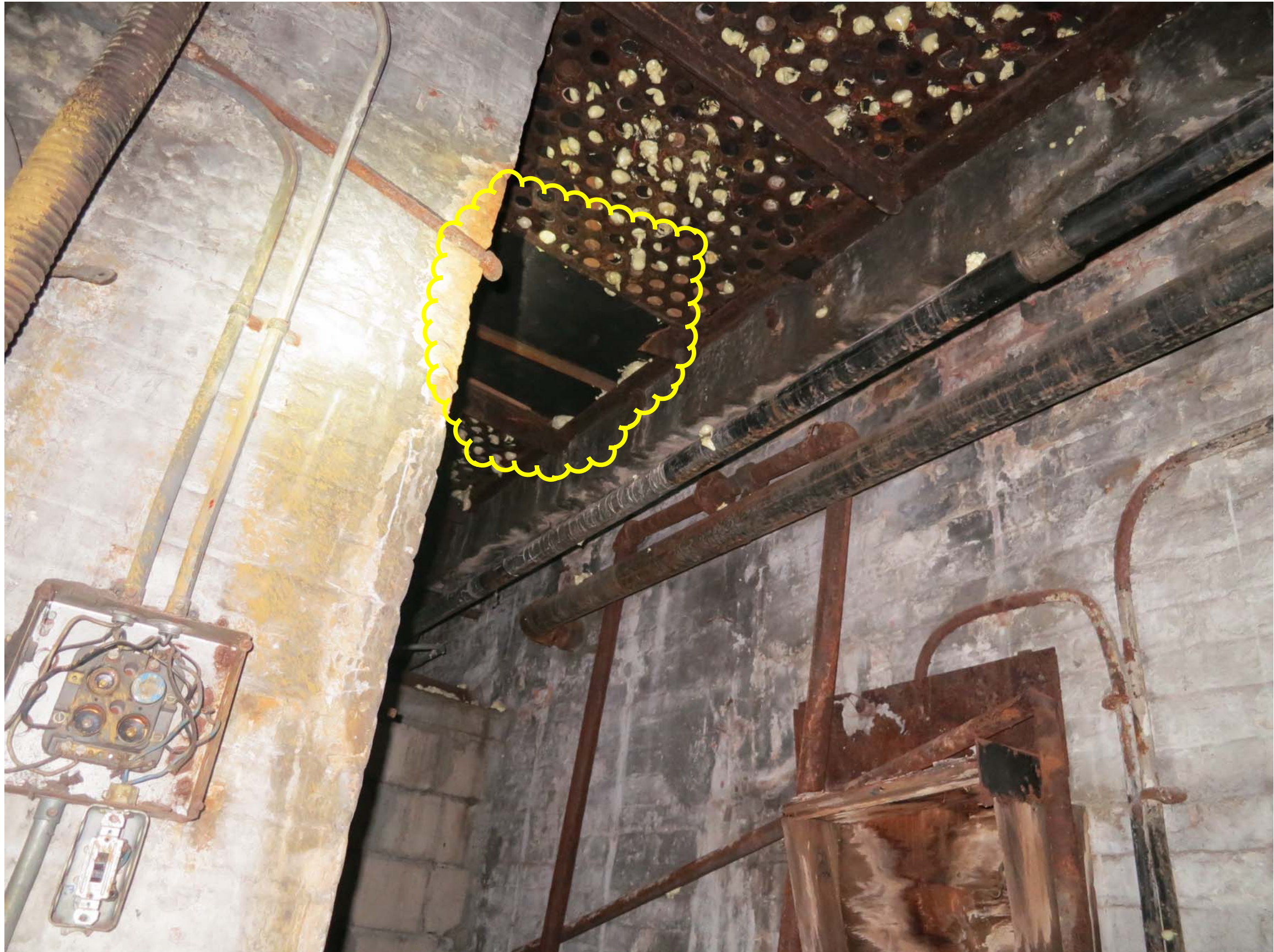
MISSING VAULT SYLIGHTS
