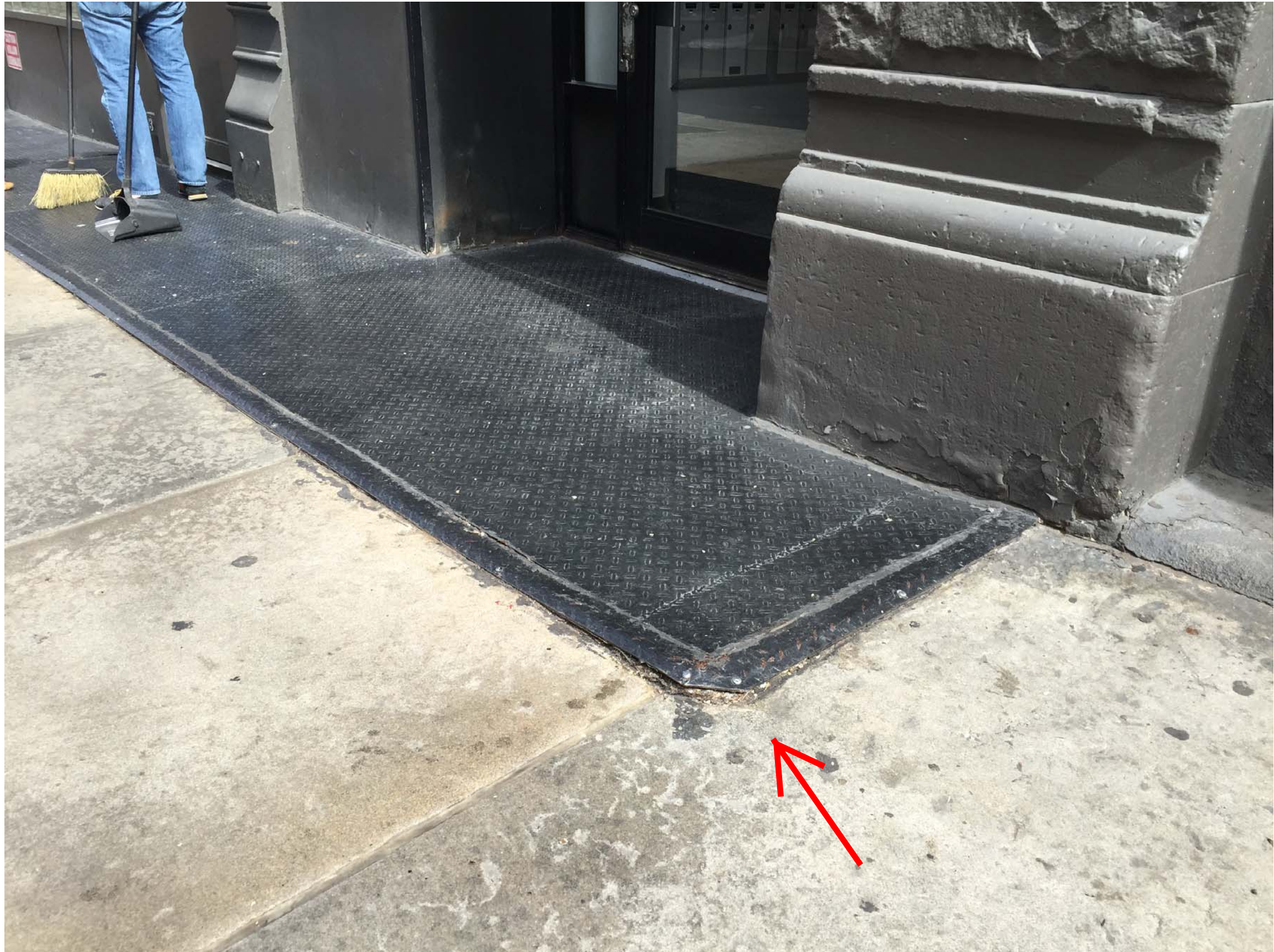
DEFECTIVE STEEL PLATES LIFTED AT THE TRIM
