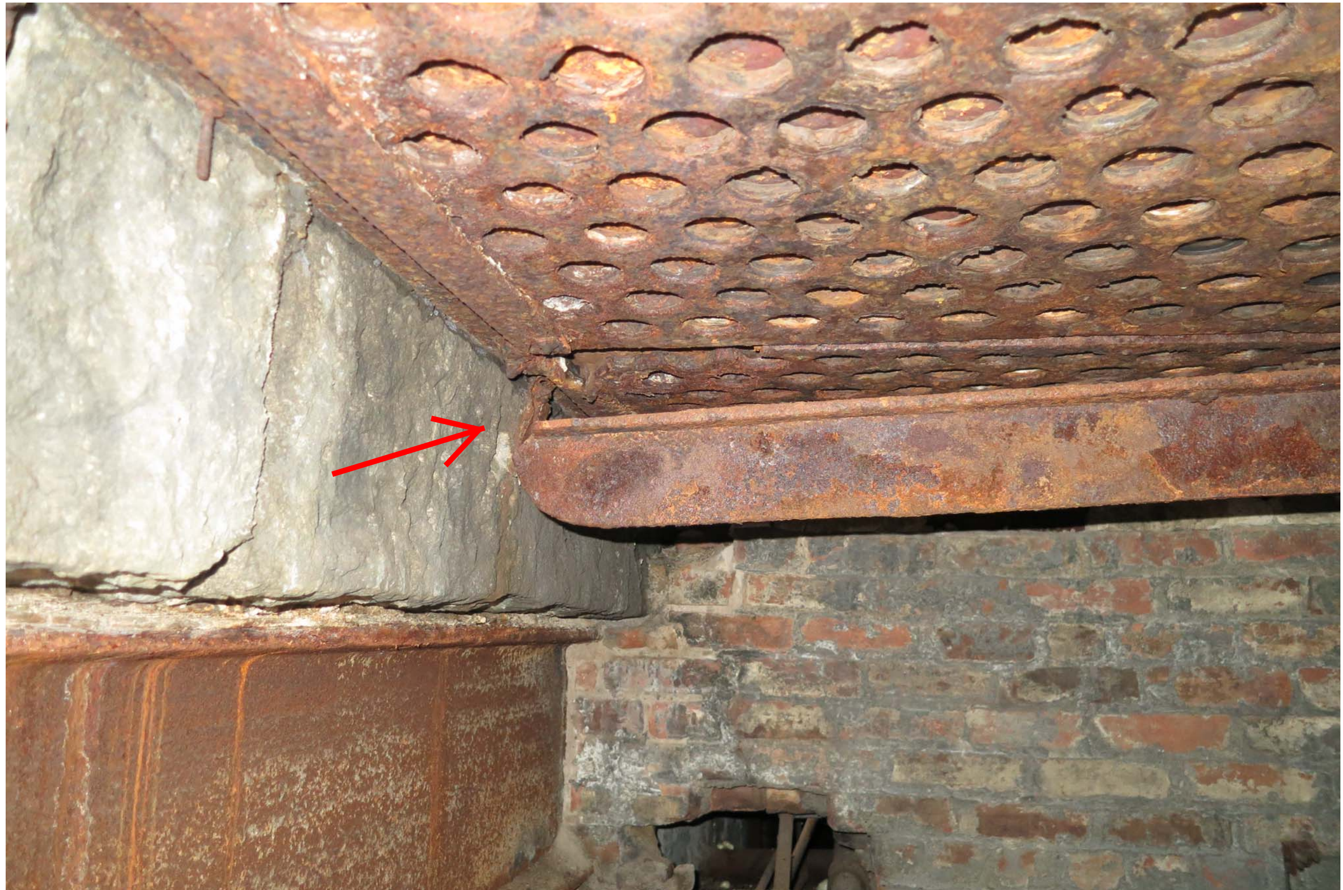
DISCONNECTED STRUCTURAL COMPONENT SUPPORTING EXISTING STEEL PLATE AND VAULT LIGHTS
