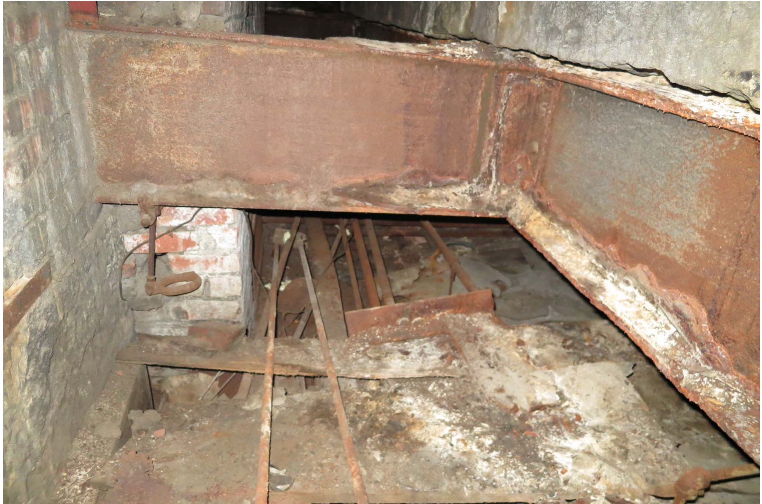
DEFECTIVE PLATING CAUSING FURTHER STRUCTURAL DAMAGE
