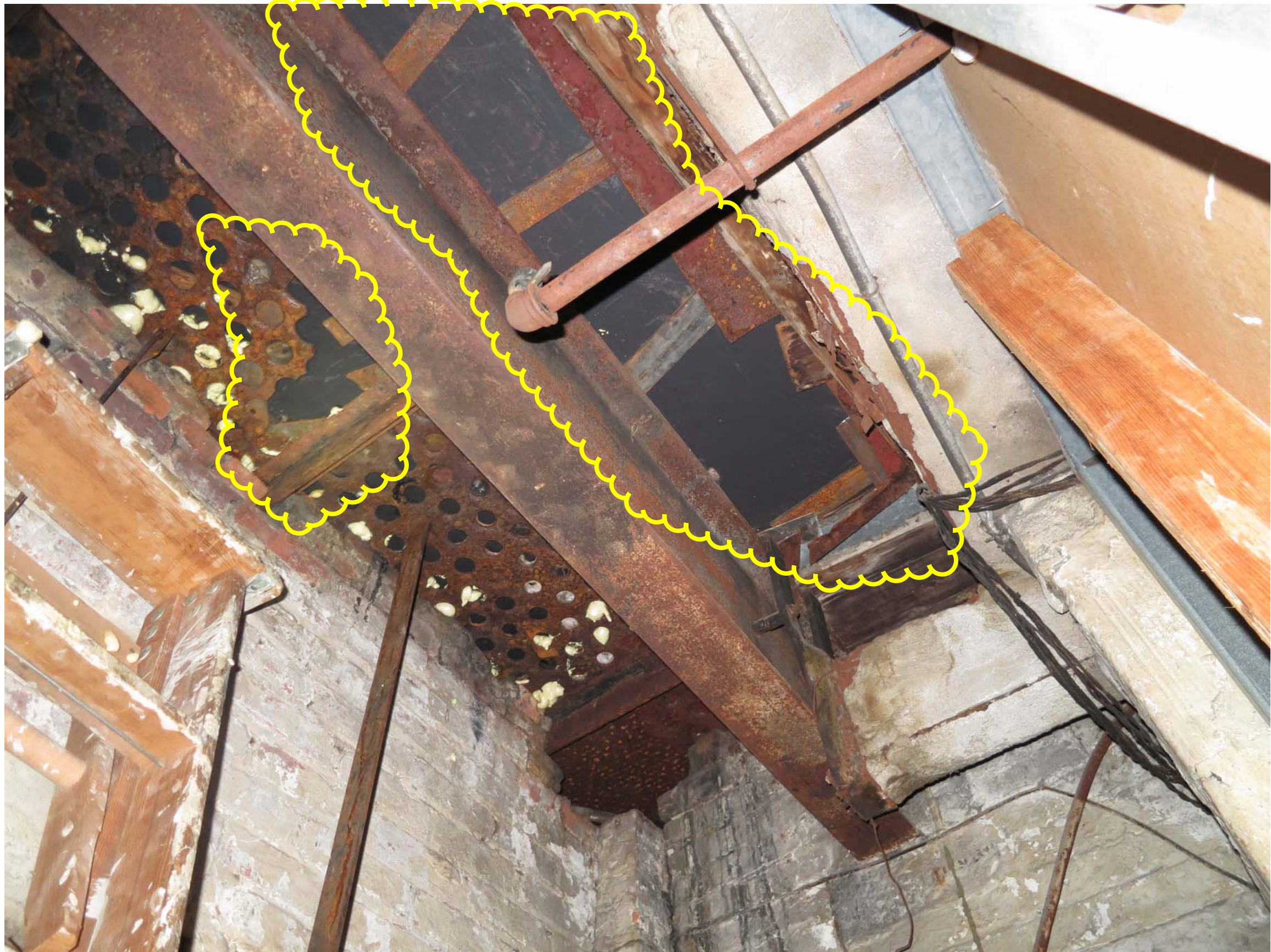
SECTIONS OF VAULT LIGHTS MISSING
