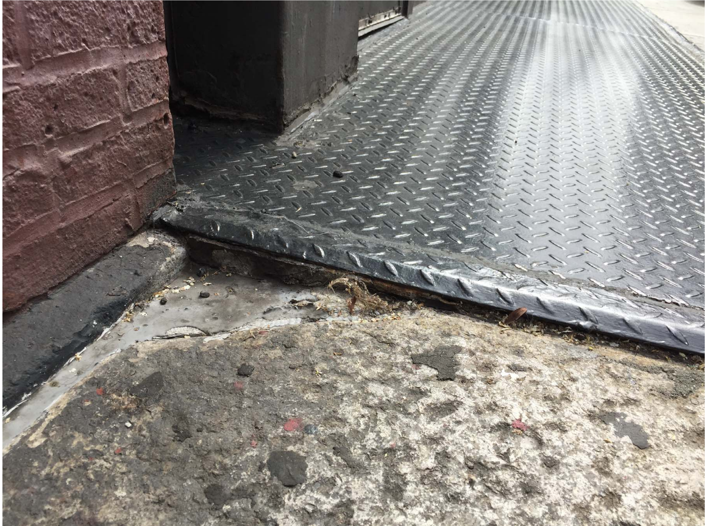
STEEL PLATE CONDITIONS AT THE PERIMETER TRIMMING
