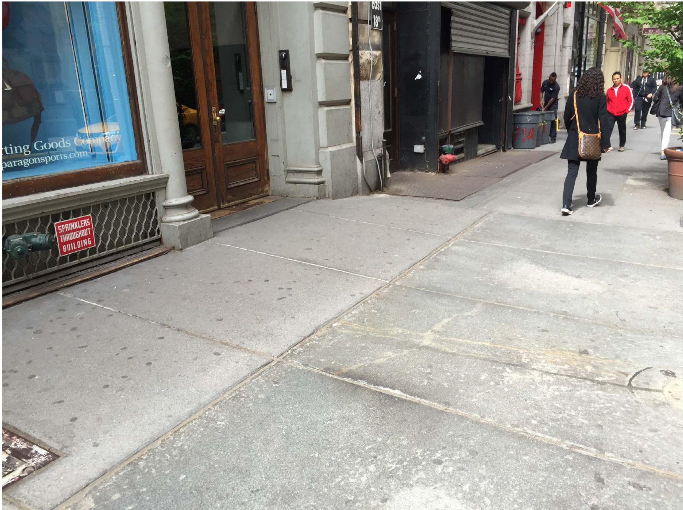
EXAMPLES OF PROPOSED CONCRETE SLAB PLACEMENT AS A CONTINUATION OF STONE SIDEWALK SLAB
