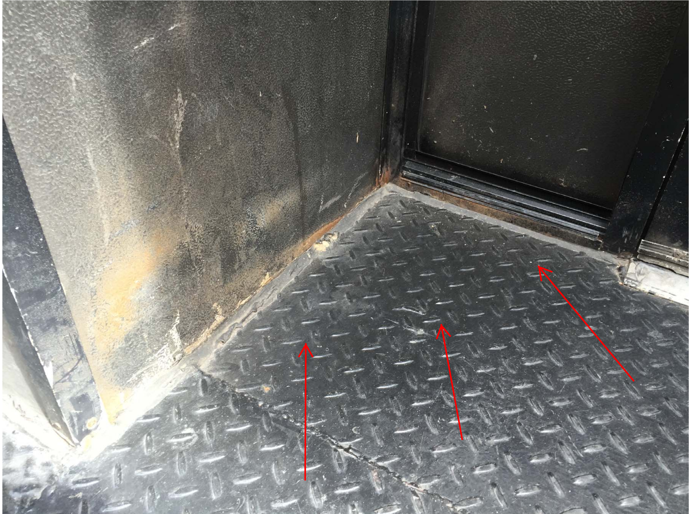
BACK PITCHED PLATING CAUSING WAER INFILTRATION INTO BUILDING ENTRANCE
