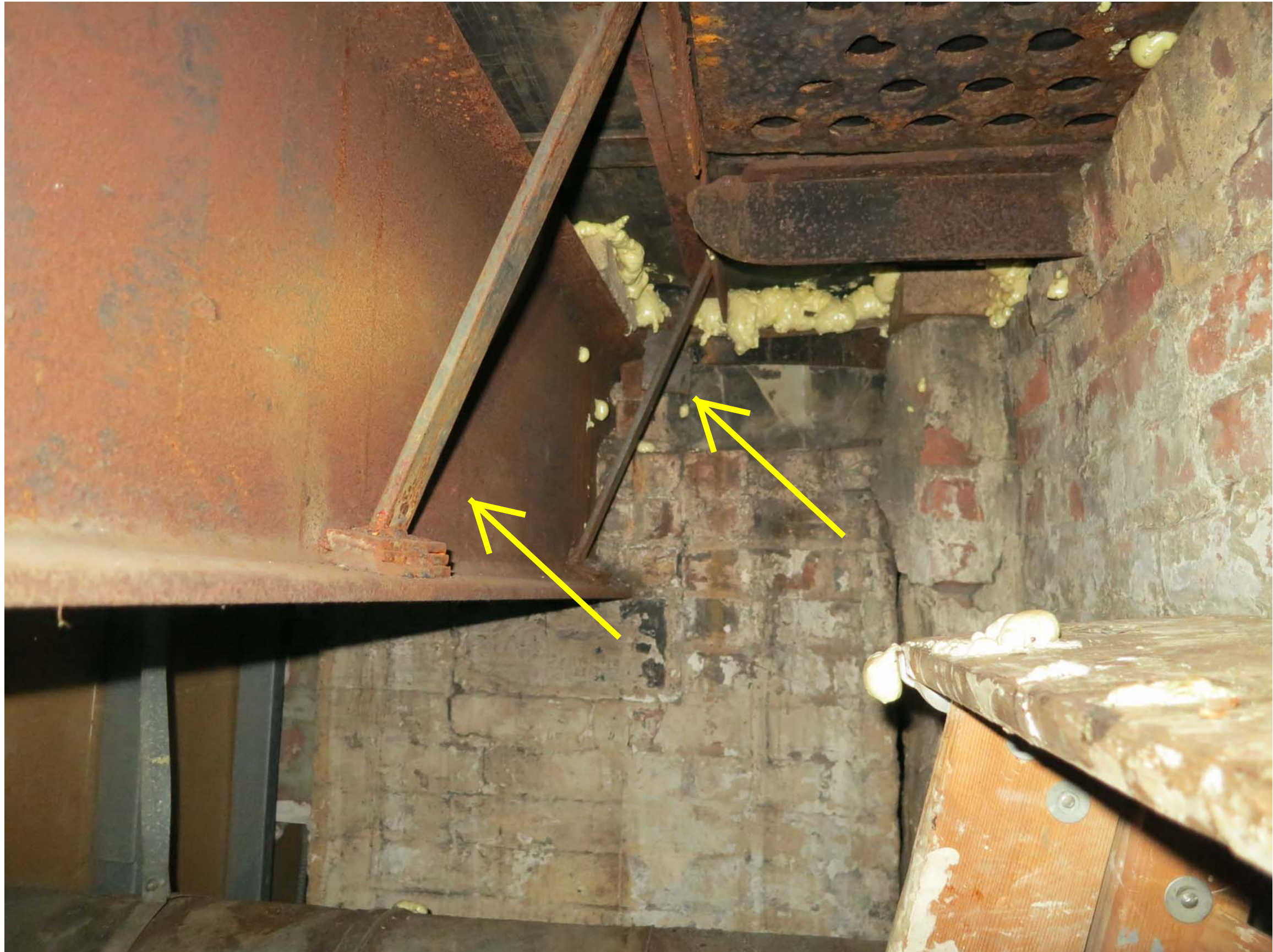
ORIGINAL STRUCTURAL FRAMING IS INADEQUATE FOR SUPPORTING THE DESIGN LOADING OVER THE STEEL PLATE
