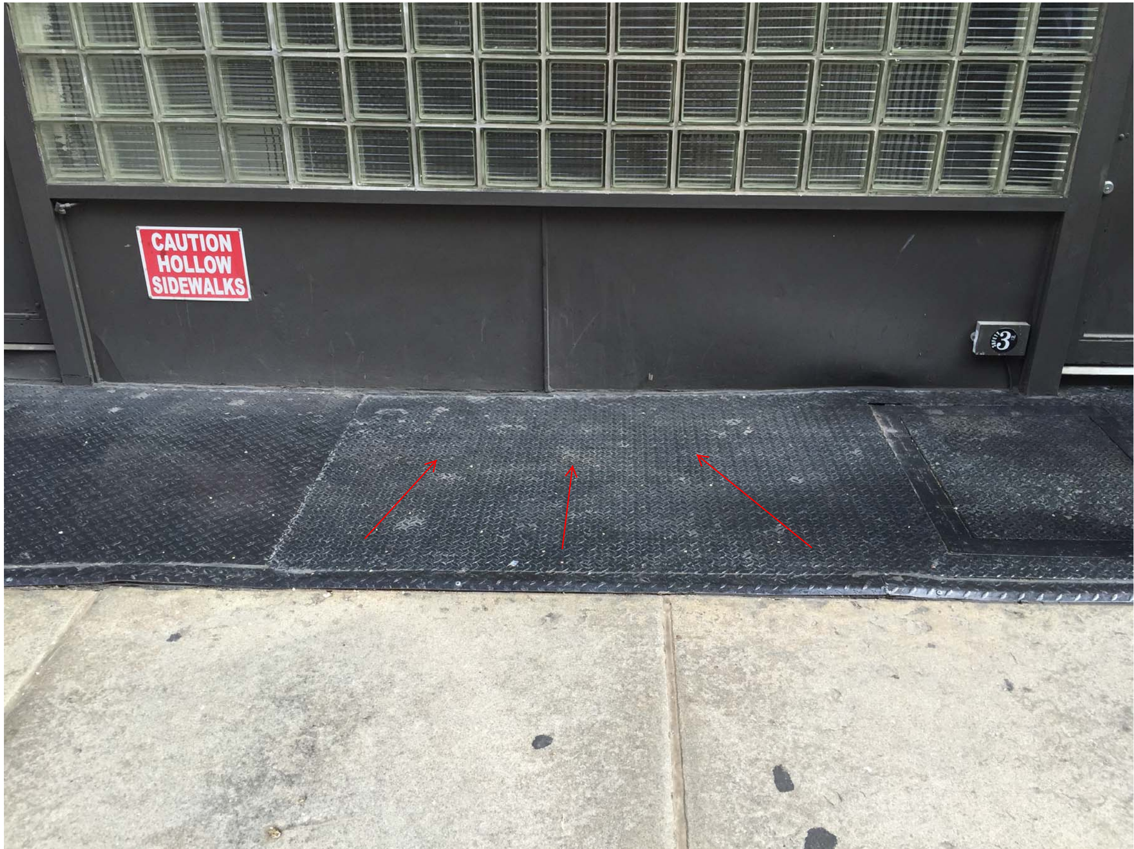
BOWED STEEL PLATING ALLOWING WATER TO POOL AND INFILTRATE
