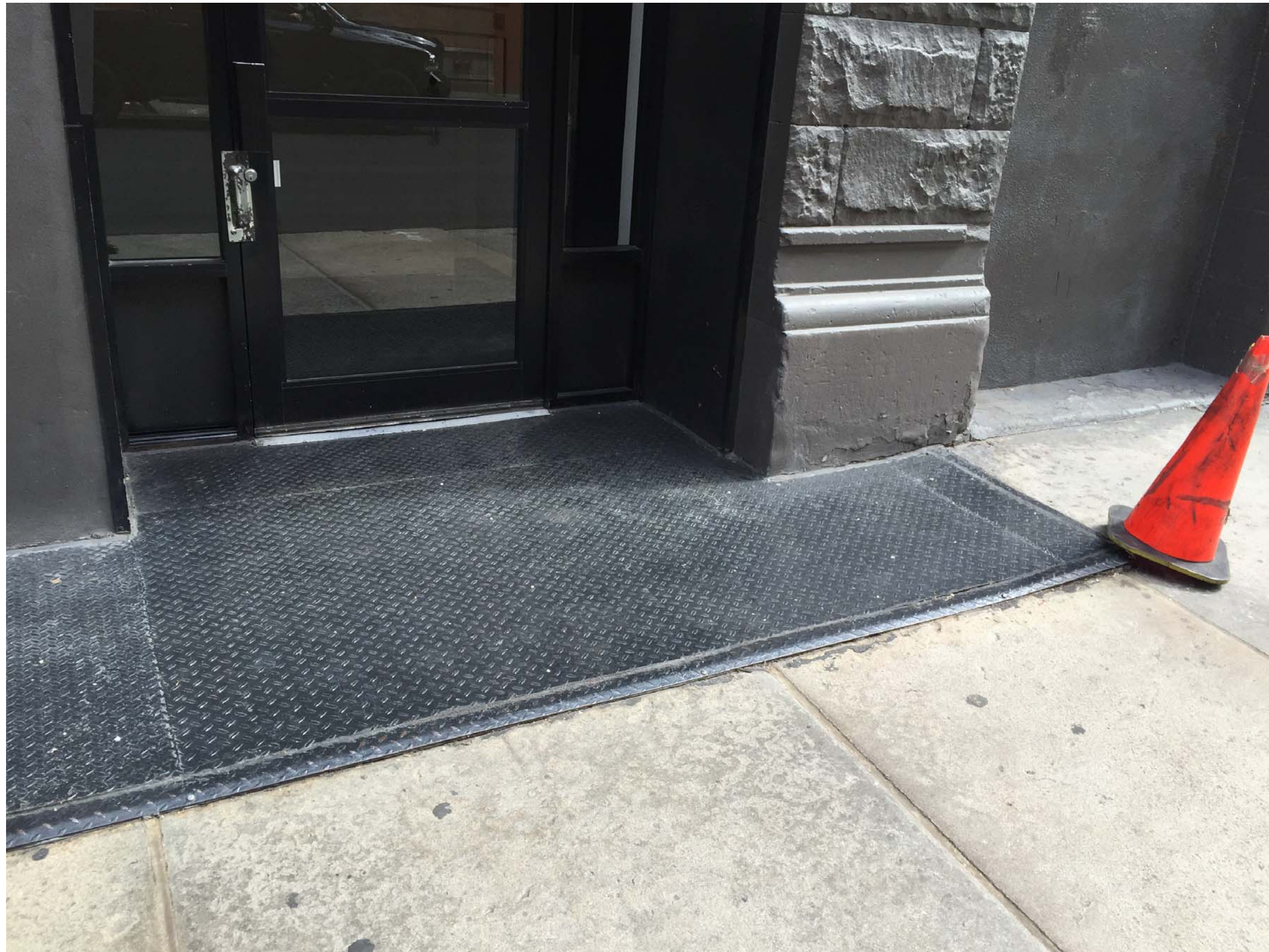
PRECAUTIONARY MEASURES FOR TRIP HAZARD CAUSED BY THE DAMAGE
