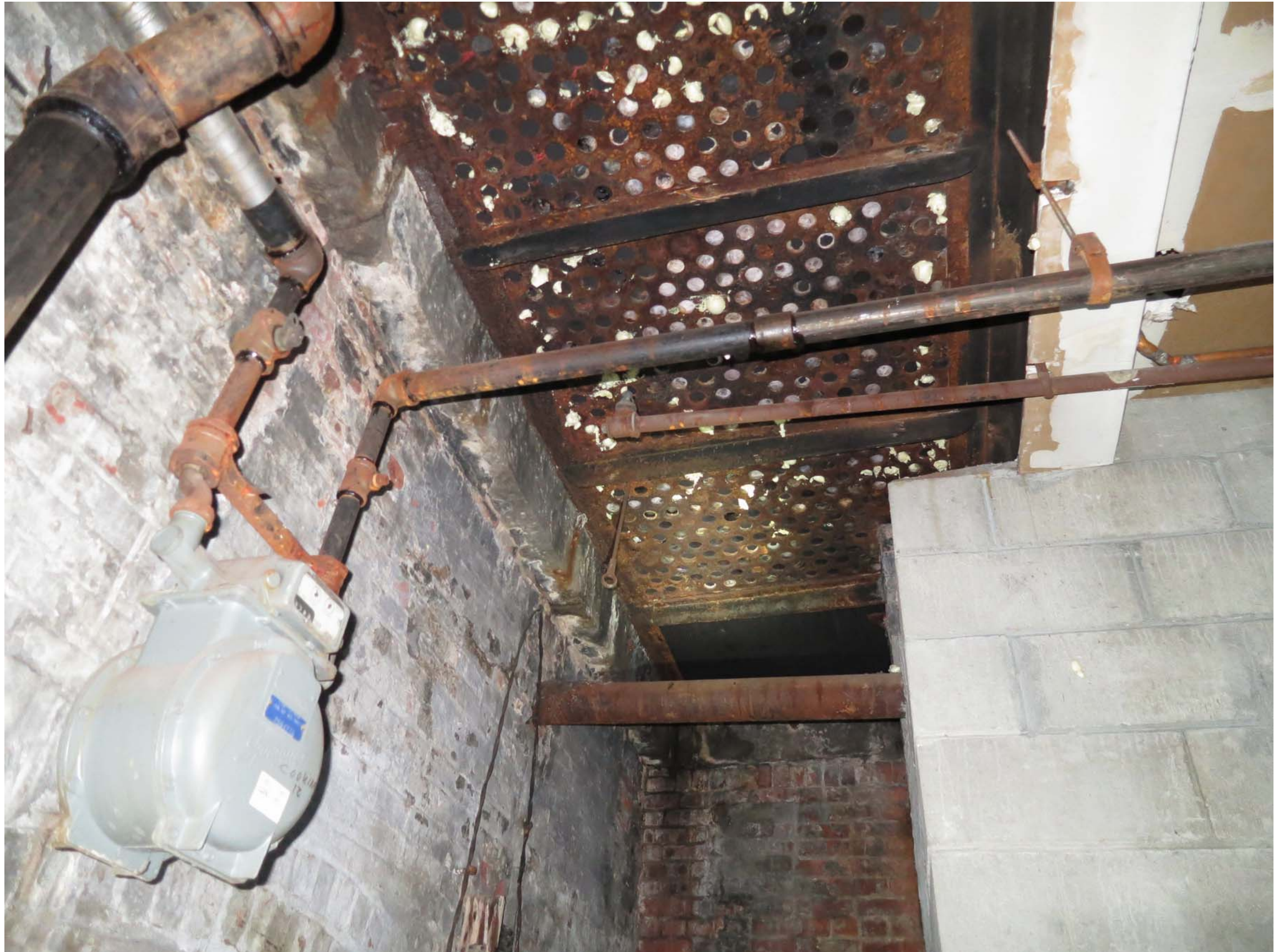
HEAVY CORROSION AFFECTING STRUCTURAL INTEGRITY
