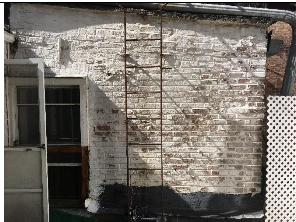
REAR FAÇADE EXTERIOR WALL SEPARATING EASTERN AND WESTERN PORTION EXHIBITING DETERIORATION AT WINDOW
