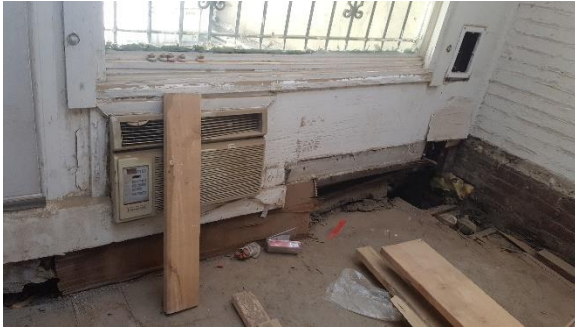
REAR EASTERN PORTION OF WOOD FRAMING, DAMAGE/DISPLACEMENT AT WALL FLOOR INTERFACE
