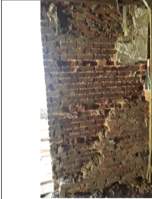
MASONRY WALL WITH EXTENSIVE LOSS OF MASONRY, ONE WYTHE COLLAPSE
