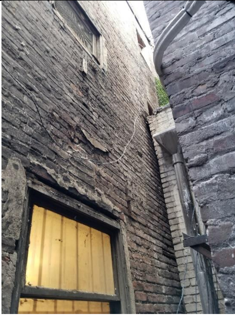
BRICKS BETWEEN TWO WINDOWS ARE WATER DAMAGED AT 275 REAR SIDE FAÇADE
