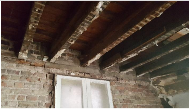
JOISTS FRAMING INTO MASONRY IN POOR CONDITION, MASONRY IN POOR CONDITION
