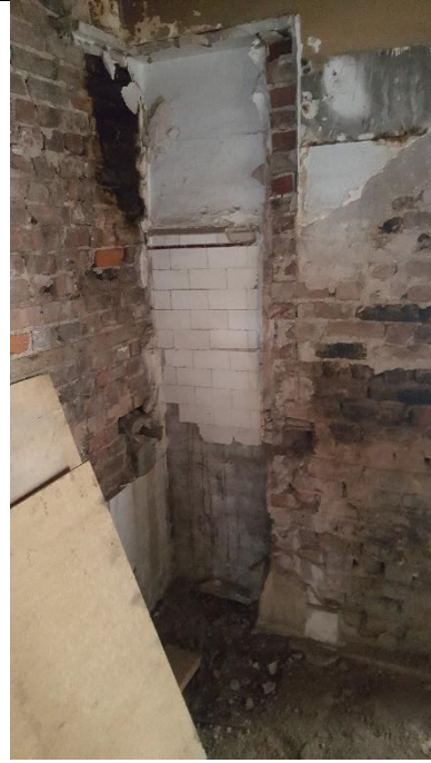
MASONRY WALL EXHIBTING DETERIORATION
