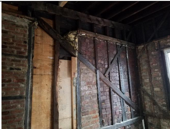
FRONT PORTION INTERIOR NOGGIN WALL EXHIBITING GAPS IN MASONRY INFILL
