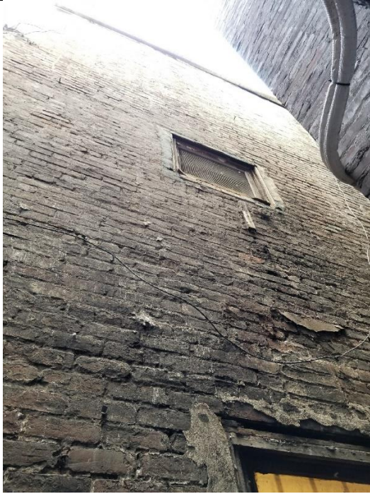
DISINTEGRATED LOOSE MORTAR BETWEEN BRICKS
