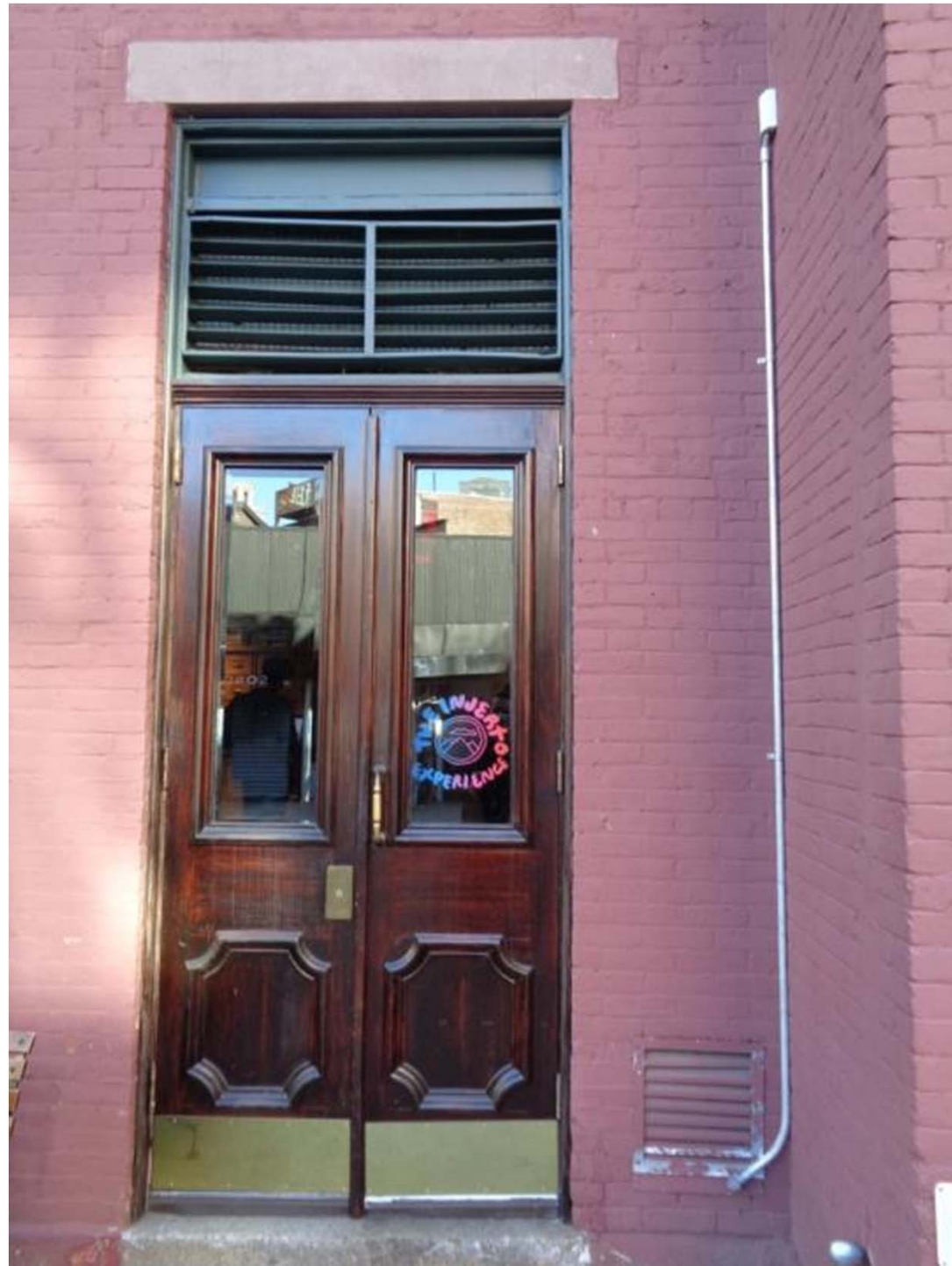
Photo 7: Current photo of the existing double door assembly along the West (MacDougal Street) facing primary facade, to be removed and replaced with a new power-assisted ADA-compliant door assembly and sidelight. Door assembly to match design of existing door in style and finish. Sidelight to match design of West 8 th Street entrance (photo 8). Existing frame, exhaust panel and blank-out panel to remain.
