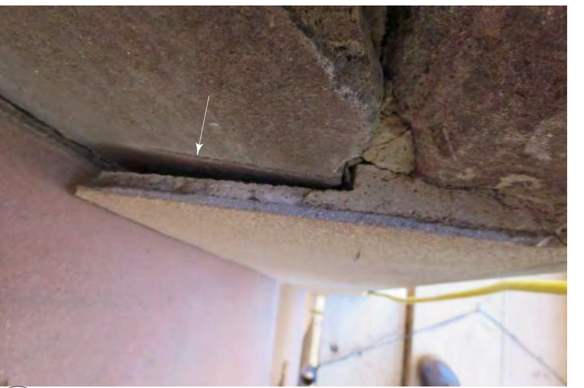
PH-14 DELAMINATED STUCCO CLOSE-UP LOOKING DOWN AT BUMP-OUT PROBE
