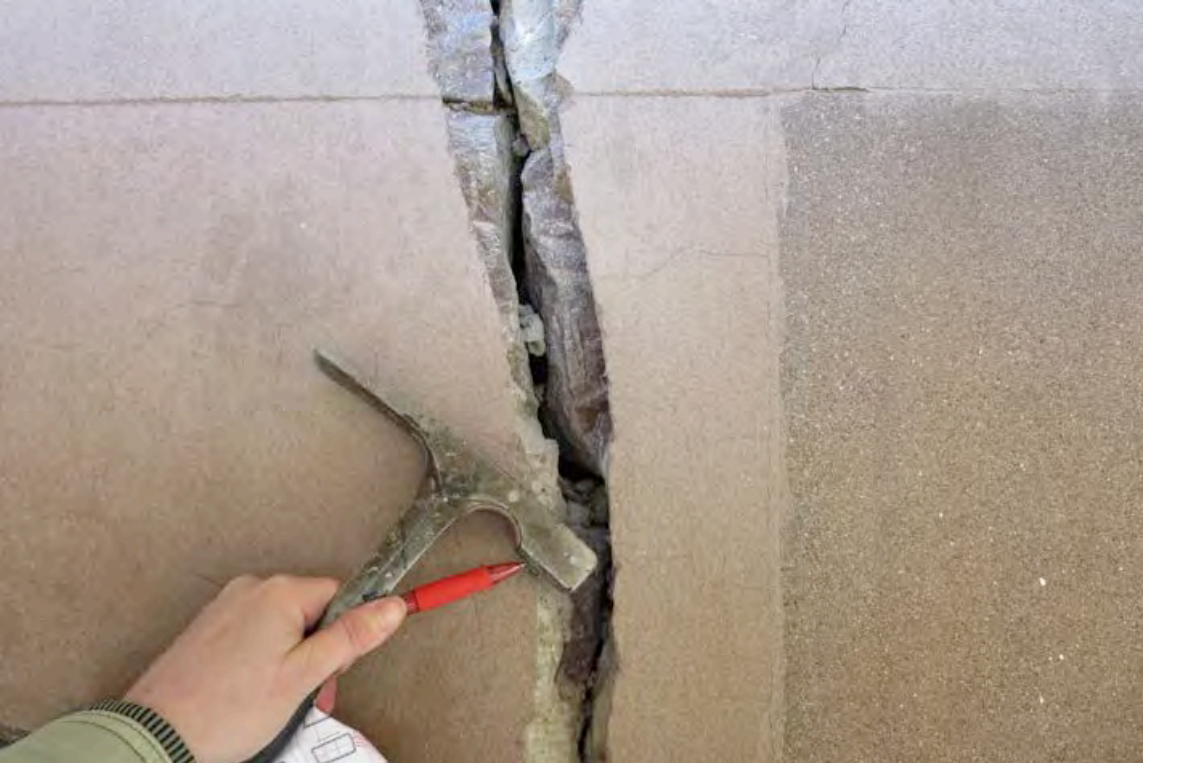
PH-12 SEVERE CRACK IN UNDERLYING BROWNSTONE BEHIND CRACKED STUCCO
