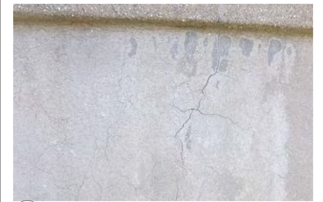
PH-9 TYPICAL HAIRLINE CRACKING BELOW WINDOW SILL
