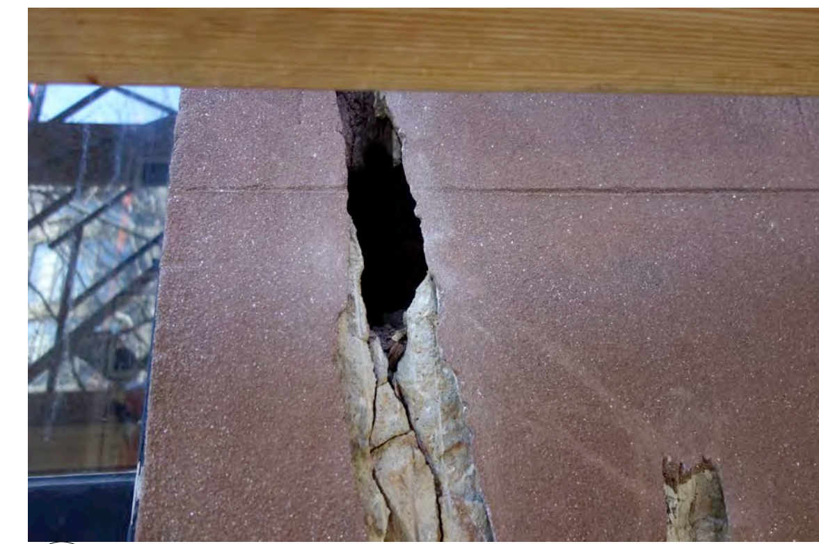
PH-6 SEVERELY DETERIORATED & MISSING MASONRY AT WINDOW JAMB WINDOW JAMB
