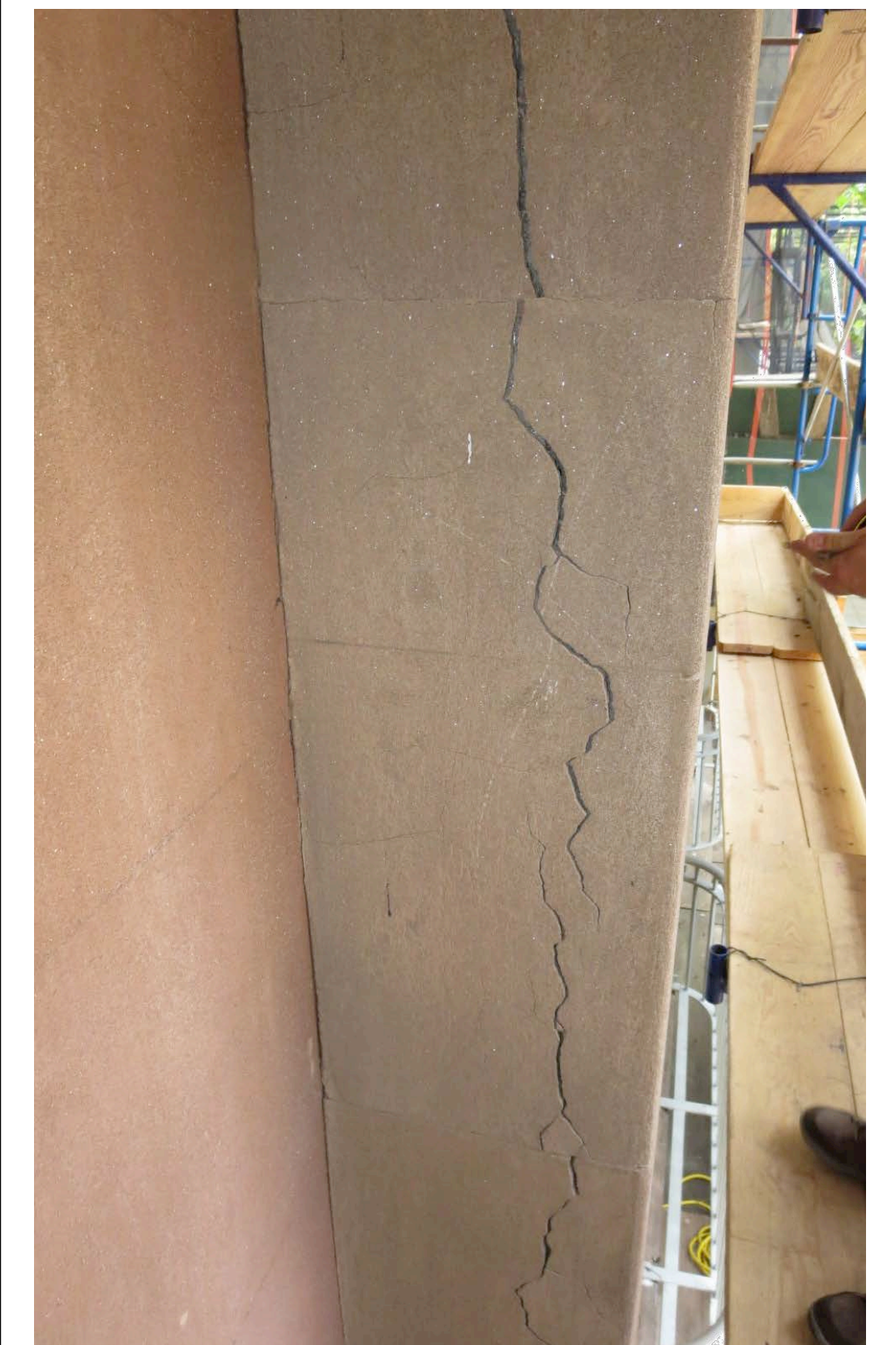
PH-13 CRACKED STUCCO BUMP-OUT BETWEEN 44 & 48 WEST 12TH STREET
