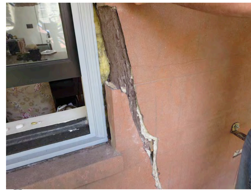
PH-5 SEVERELY DETERIORATED & MISSING MASONRY WINDOW JAMB
