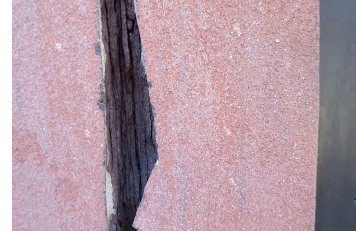
PH-4 DELAMINATING UNDERLYING MASONRY AT WINDOW JAMB WINDOW JAMB
