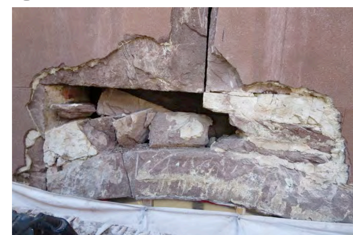
PH-8 COLLAPSED BROWNSTONE AT PANEL BETWEEN 3RD & 4TH FLOOR WINDOWS
