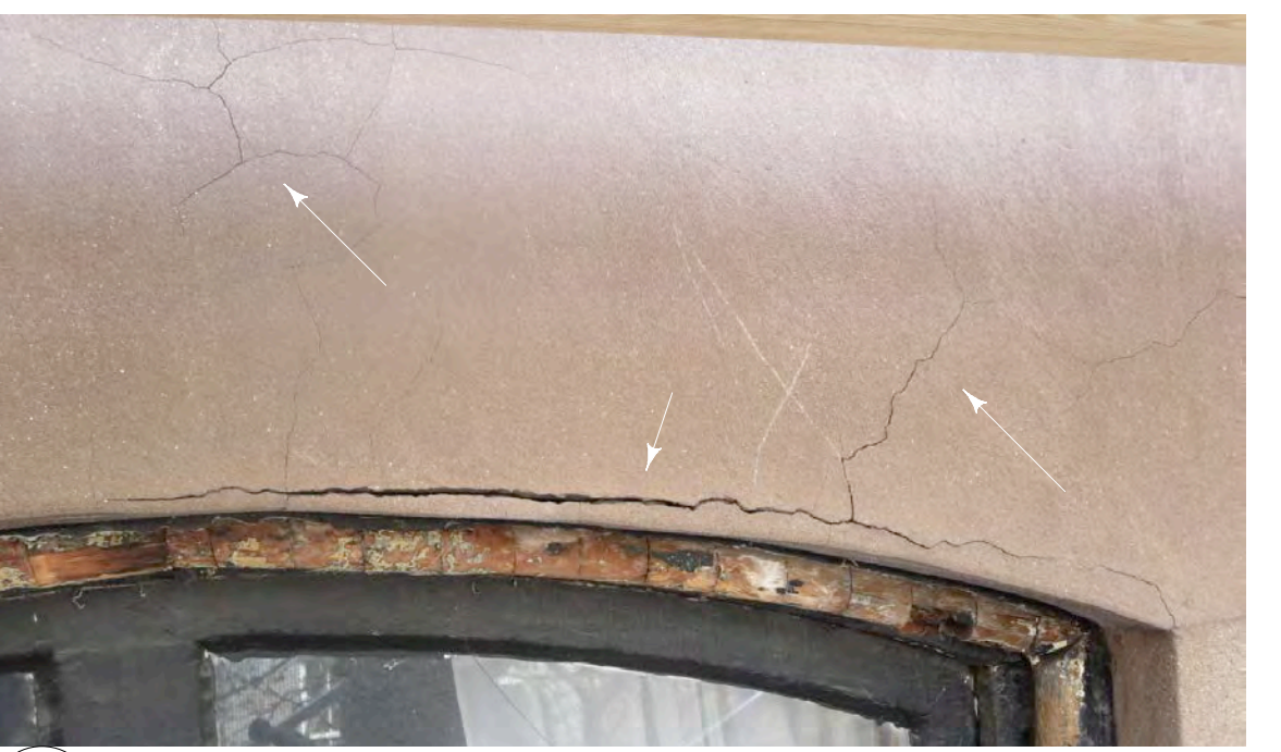
PH-10 CRACKING AT LINTEL
