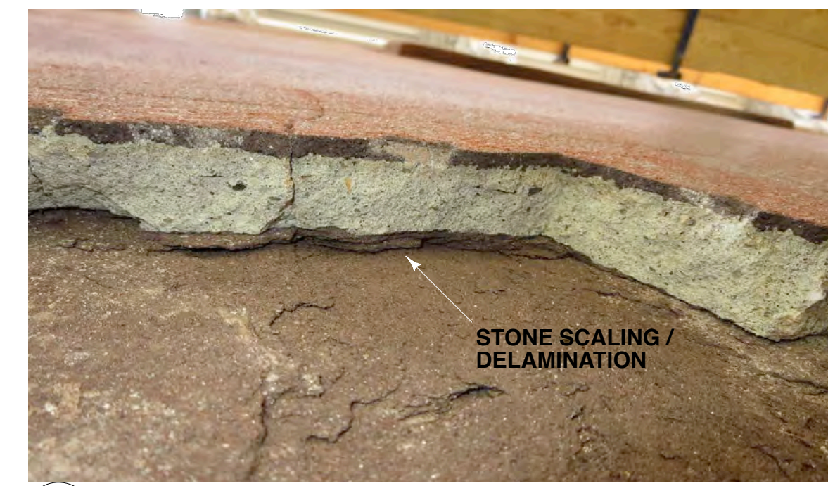
PH-2 SCALING / DELAMINATING BROWNSTONE UNDER STUCCO CLOSE-UP AT PROBE
