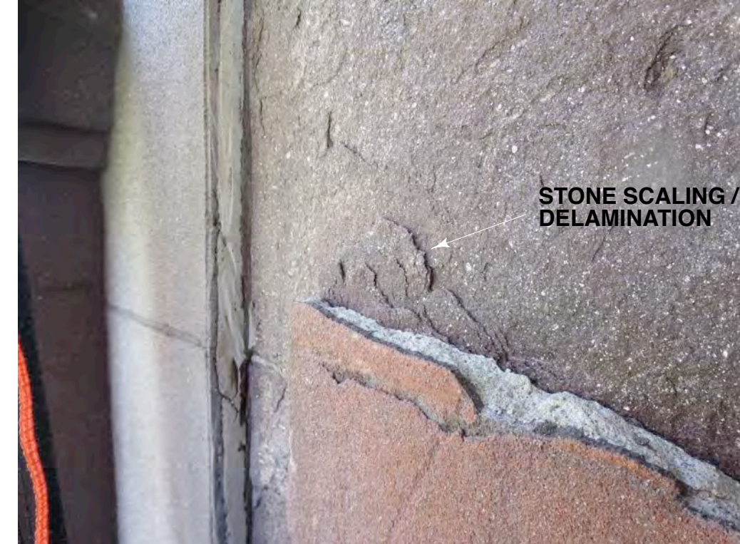
PH-3 SCALING / DELAMINATING BROWNSTONE UNDER STUCCO CLOSE-UP AT PROBE
