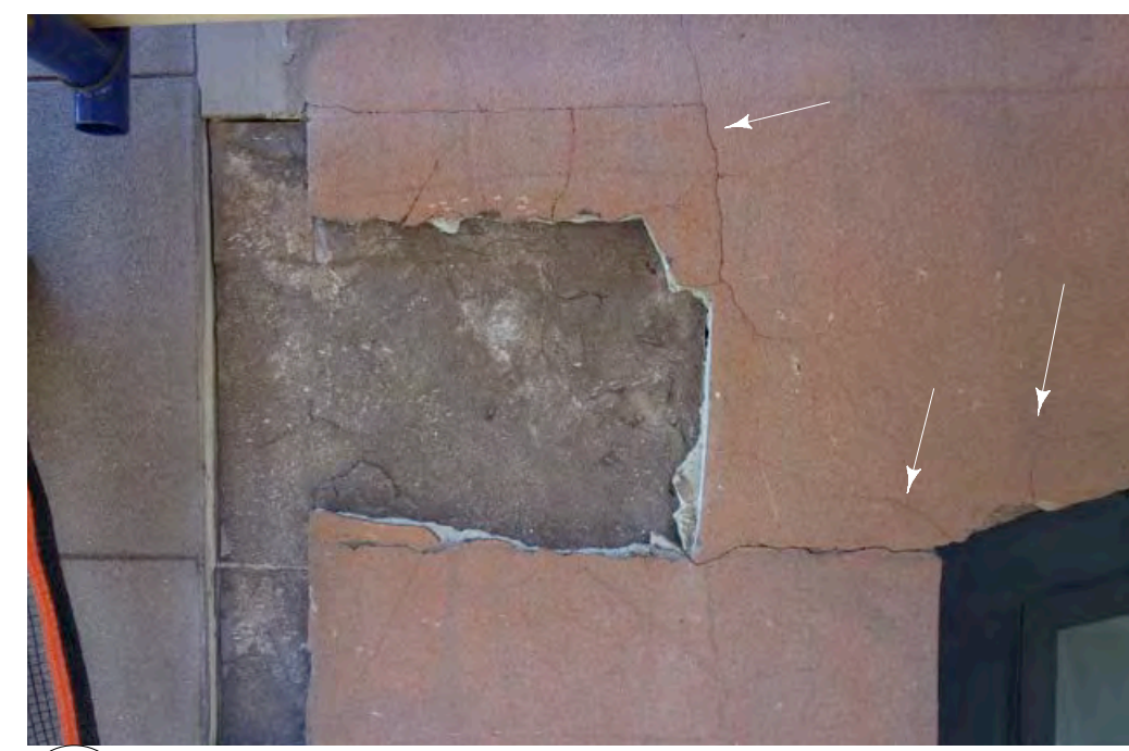
PH-1 HAIRLINE CRACKING PROBE AT EAST SIDE OF BUILDING
