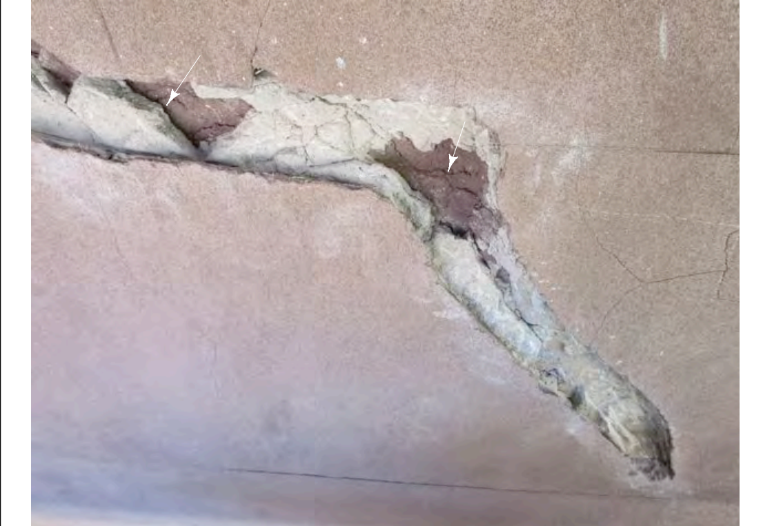
PH-11 DELAMINATING STUCCO & SCALING BROWNSTONE BEHIND CRACKED STUCCO
