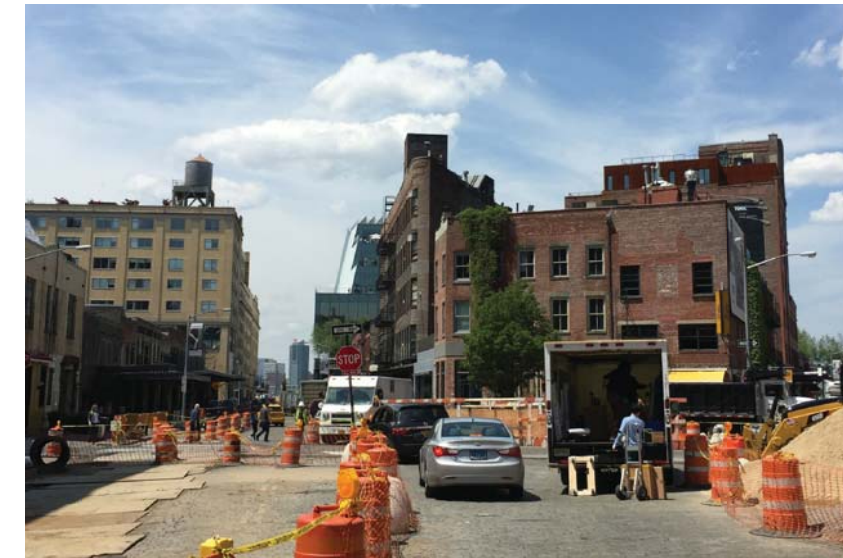
3 existing view from gansevoort st between 9th ave and hudson st n.t.s.
