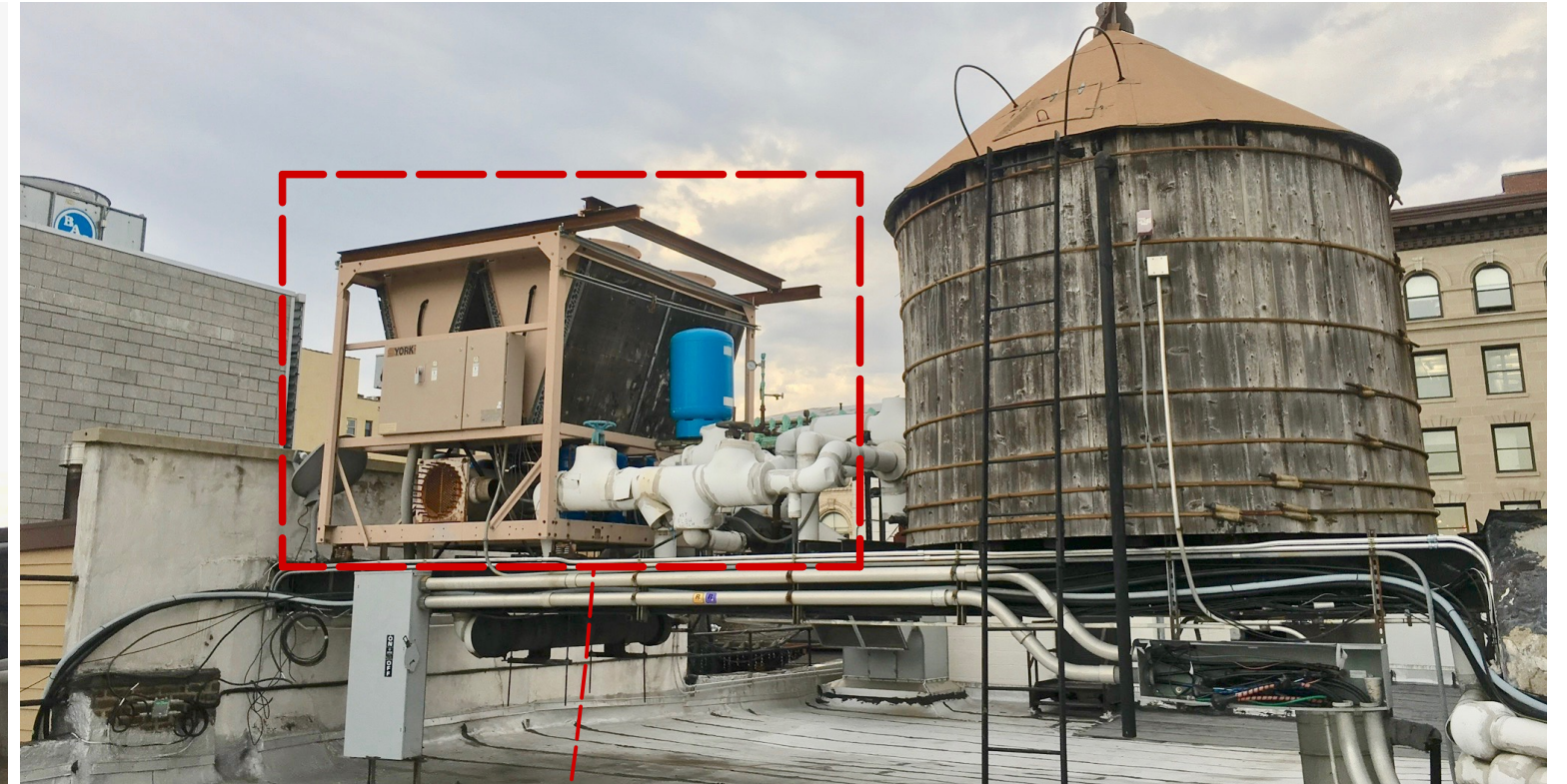
SOUTH - CHILLER UNIT
