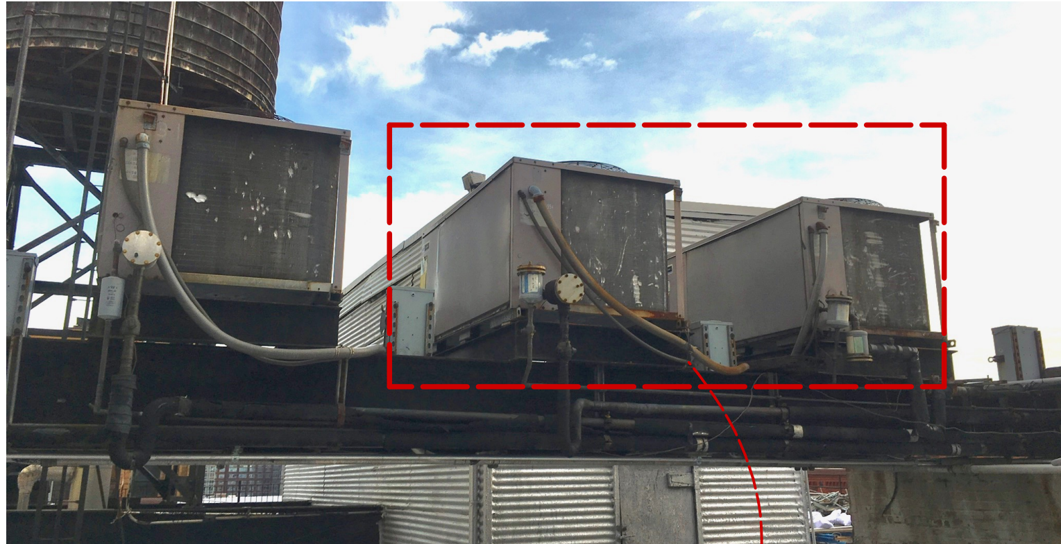
NORTH - CONDENSING UNITS
