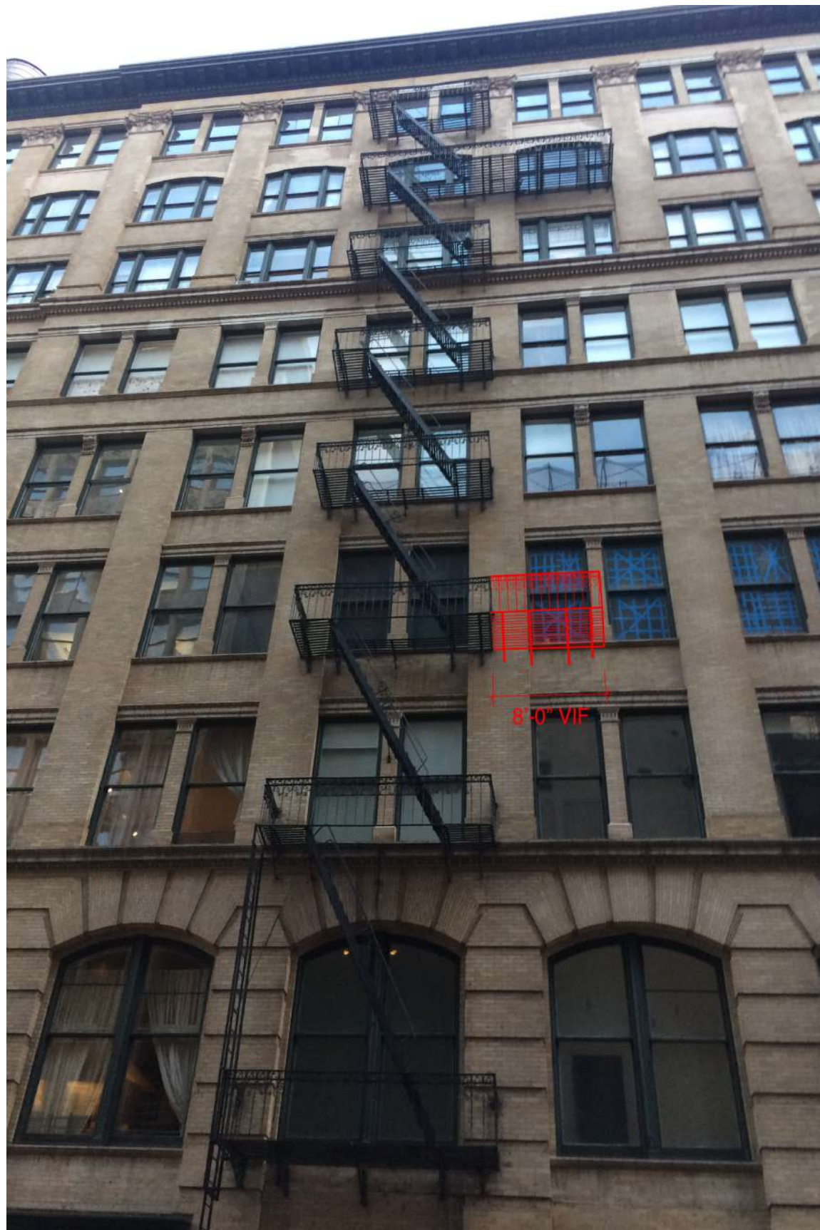
Fig. 6: 4th floor East fire escape proposed extension as seen from the street.
