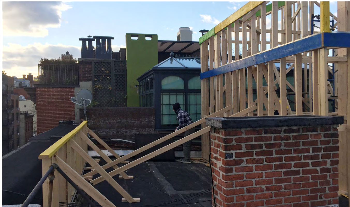
81 CHARLES ST - MOCK UP - ROOF VIEW 1 (LOOKING NORTH WEST @ RAILING, RAISED DECK & STAIR BULKHEAD)
