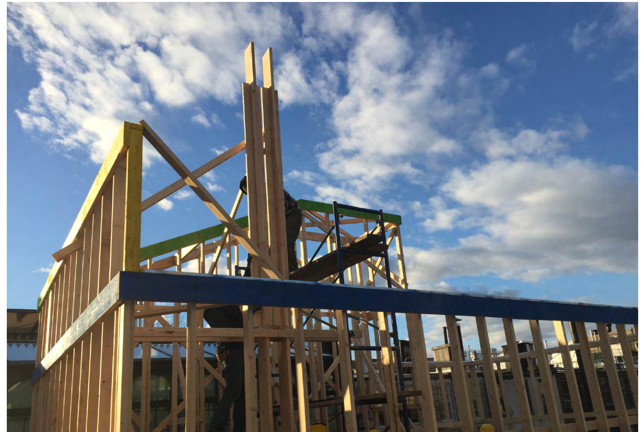
81 CHARLES ST - MOCK UP - ROOF VIEW 4 (LOOKING NORTH WEST @ FLUES, RAILING AND STAIR BULKHEAD)
