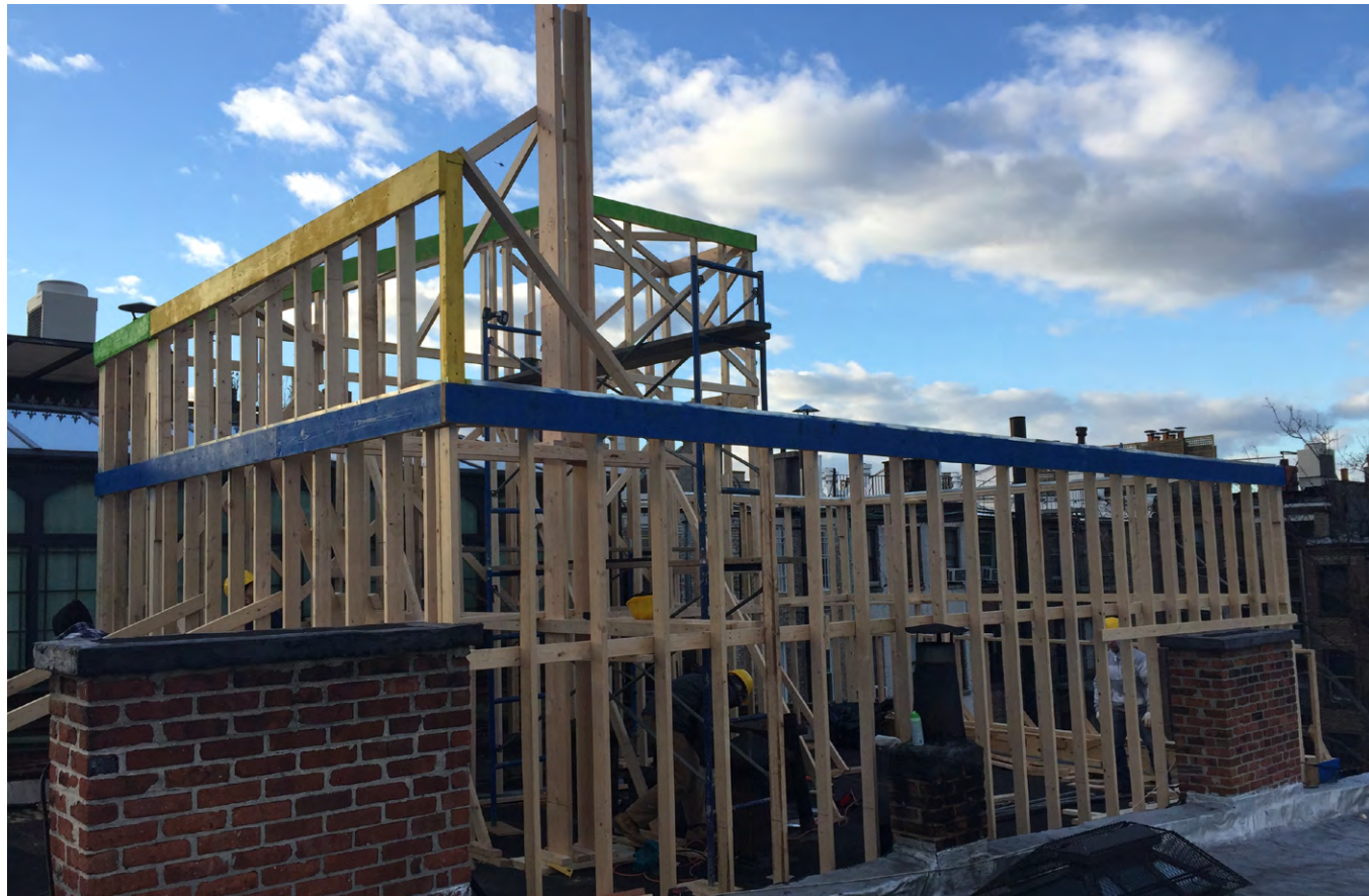
81 CHARLES ST - MOCK UP - ROOF VIEW 3 (LOOKING NORTH WEST @ EXTENT OF MOCK UP)
