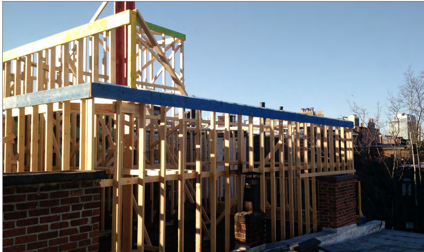
81 CHARLES ST - MOCK UP - ROOF VIEW 1 (LOOKING NORTH WEST @ RAILING, ADDITION & STAIR BULKHEAD)
