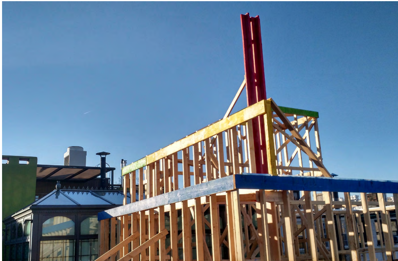
81 CHARLES ST - MOCK UP - ROOF VIEW 3 (LOOKING NORTH WEST @ EXTENT OF MOCK UP + FLUES)
