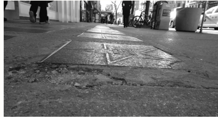
Many of the stars on the Yiddish Walk of Fame have suffered cracks and deterioration.
