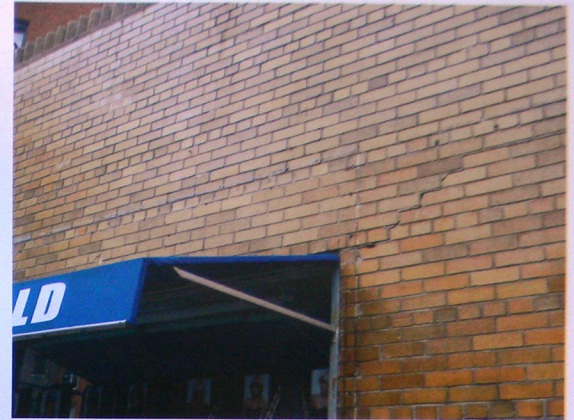
2 Cracking at Awning on 7th Av South Side
