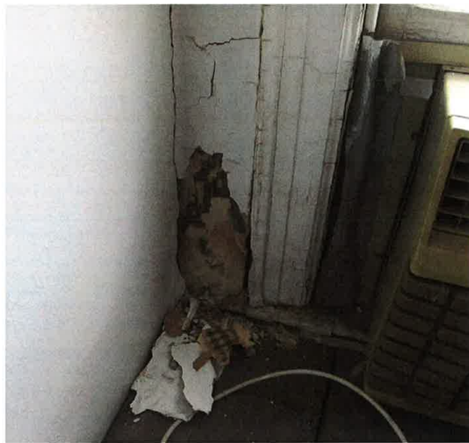
6 TYPICAL PLASTER DETERIORATION (INTERIOR SOUTH WALL) A-5
