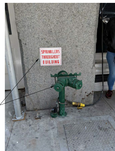
EXISTING STANDPIPE AND SIGNAGE
