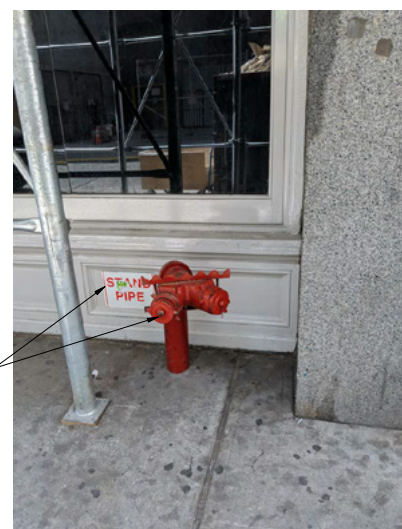
EXISTING STANDPIPE AND SIGNAGE
