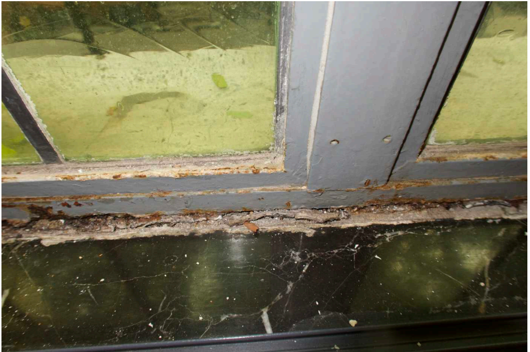
Window 4, hinges and frames rusting.
