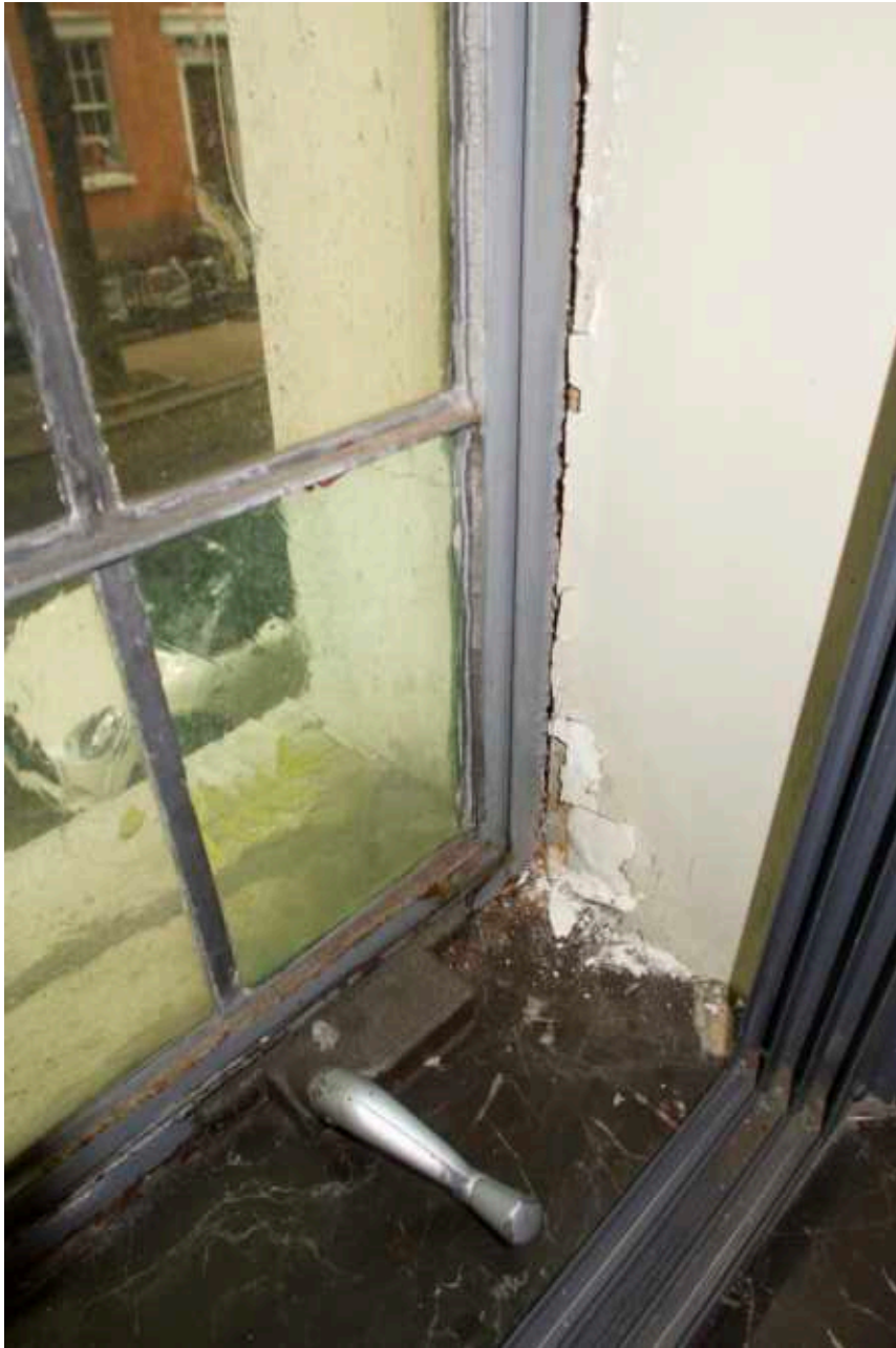
Window 2, plaster damage and rust.
