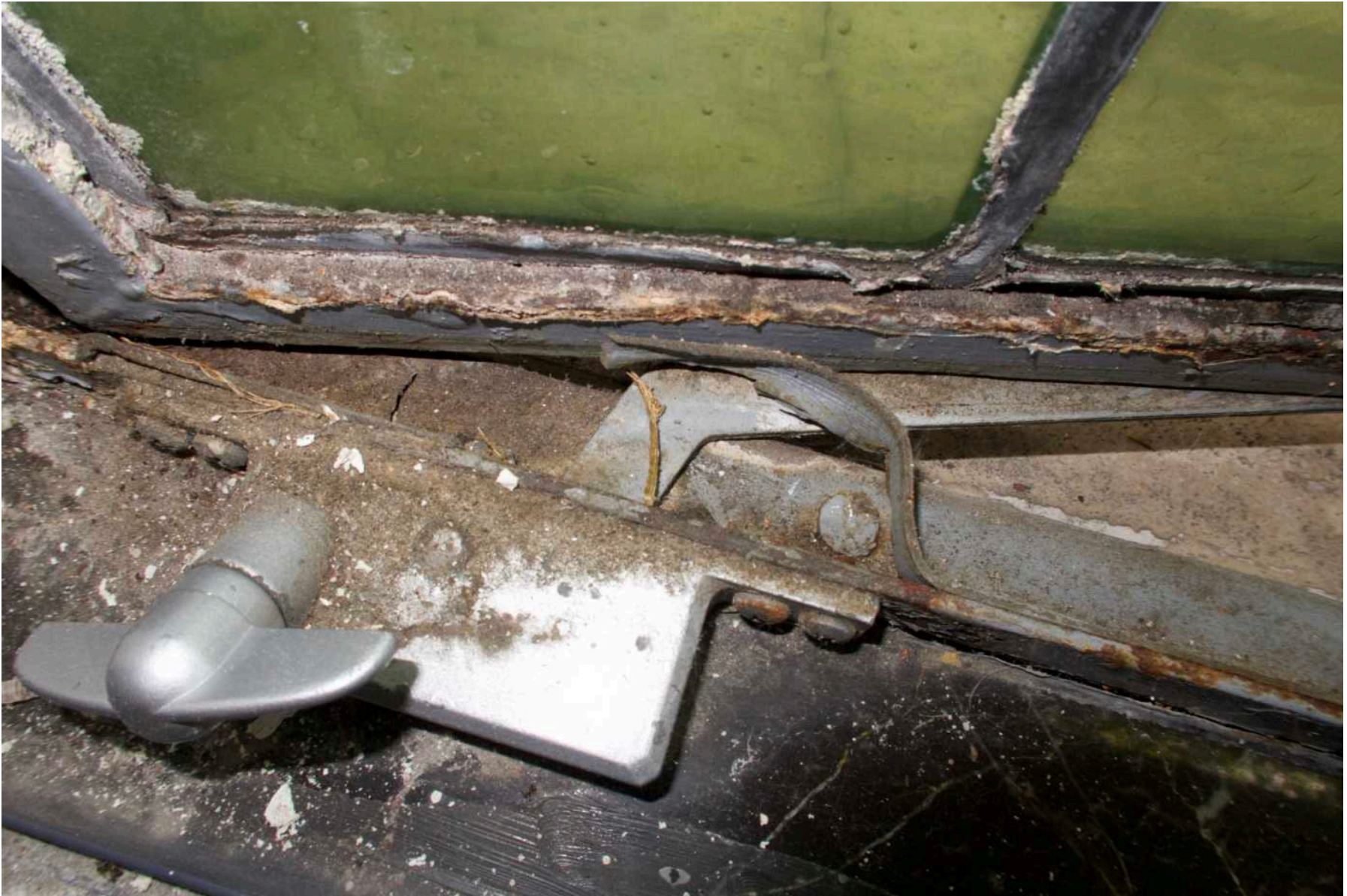
Window 5, hinge, frame rusting, insulation failure.
