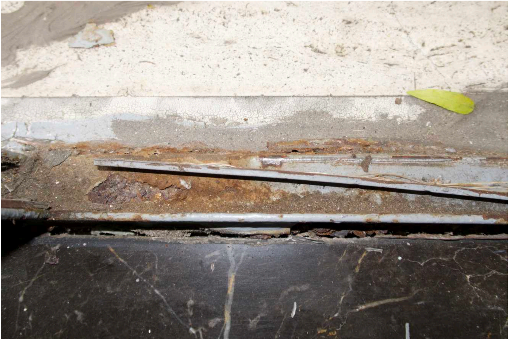
Window 3 and others, universal frames and hinges damages.
