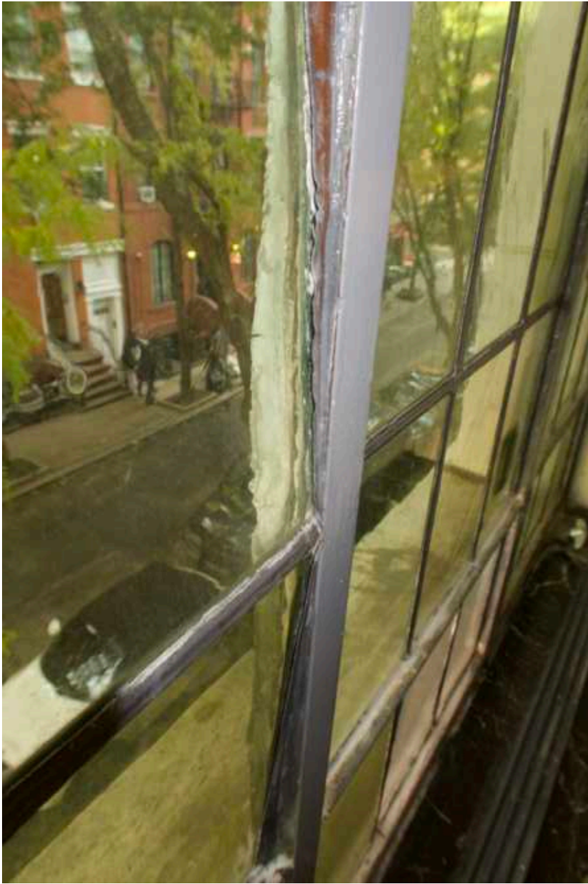
Window 5, bowing and buckling.
