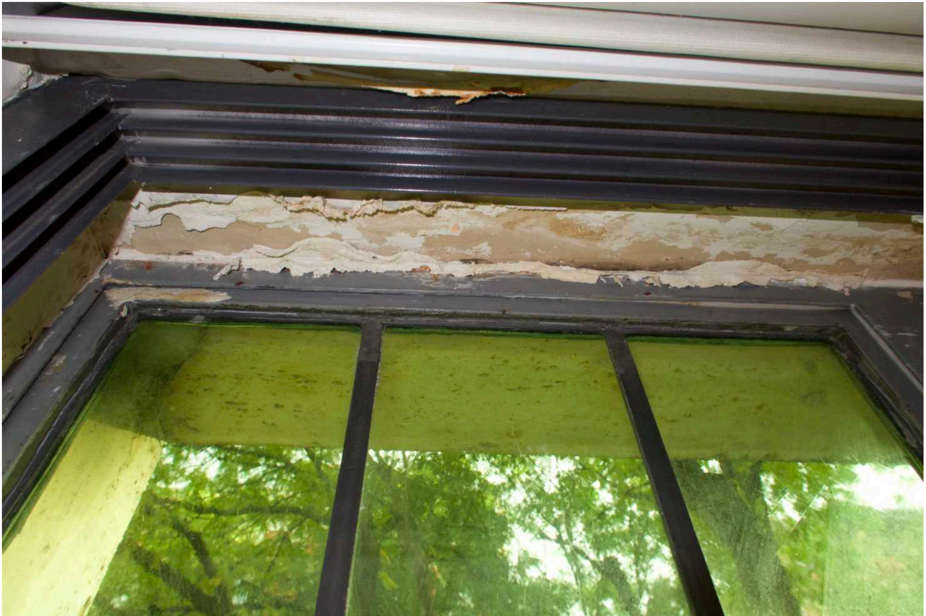
Window 4, severe top plaster damage.
