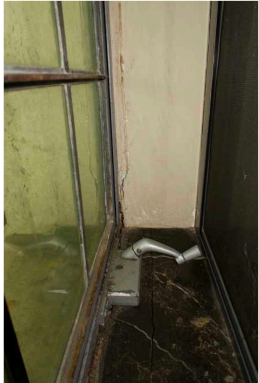
Window 3, plaster damage and rust.
