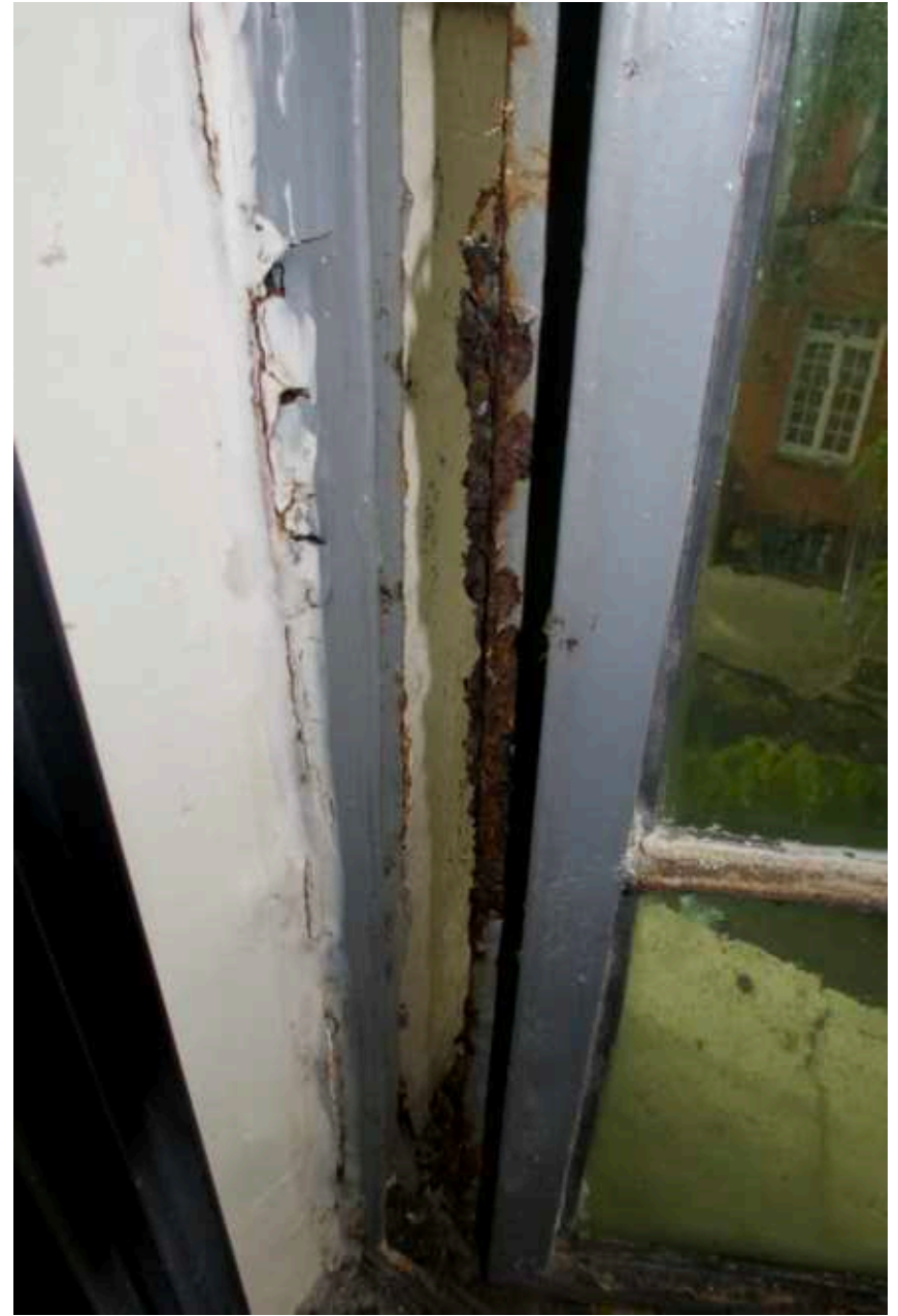
Window 5, frames rusting.
