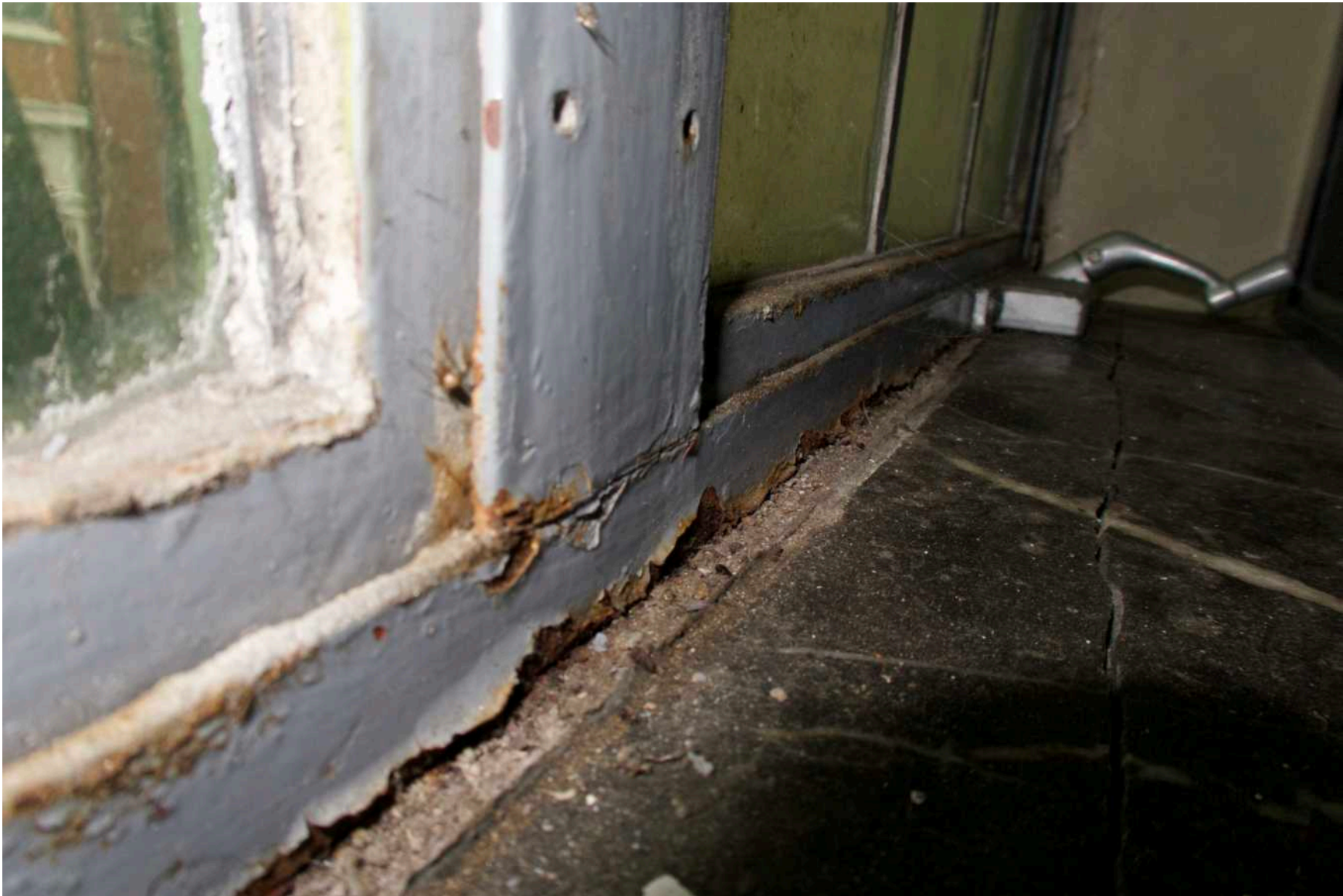
Window 2 and others, universal frames and marble damages.
