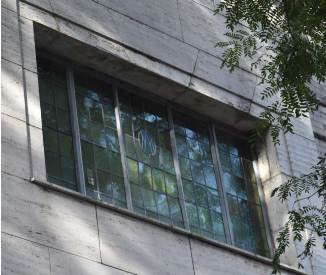
Figure 16: Window 5, Exterior, deflection.
