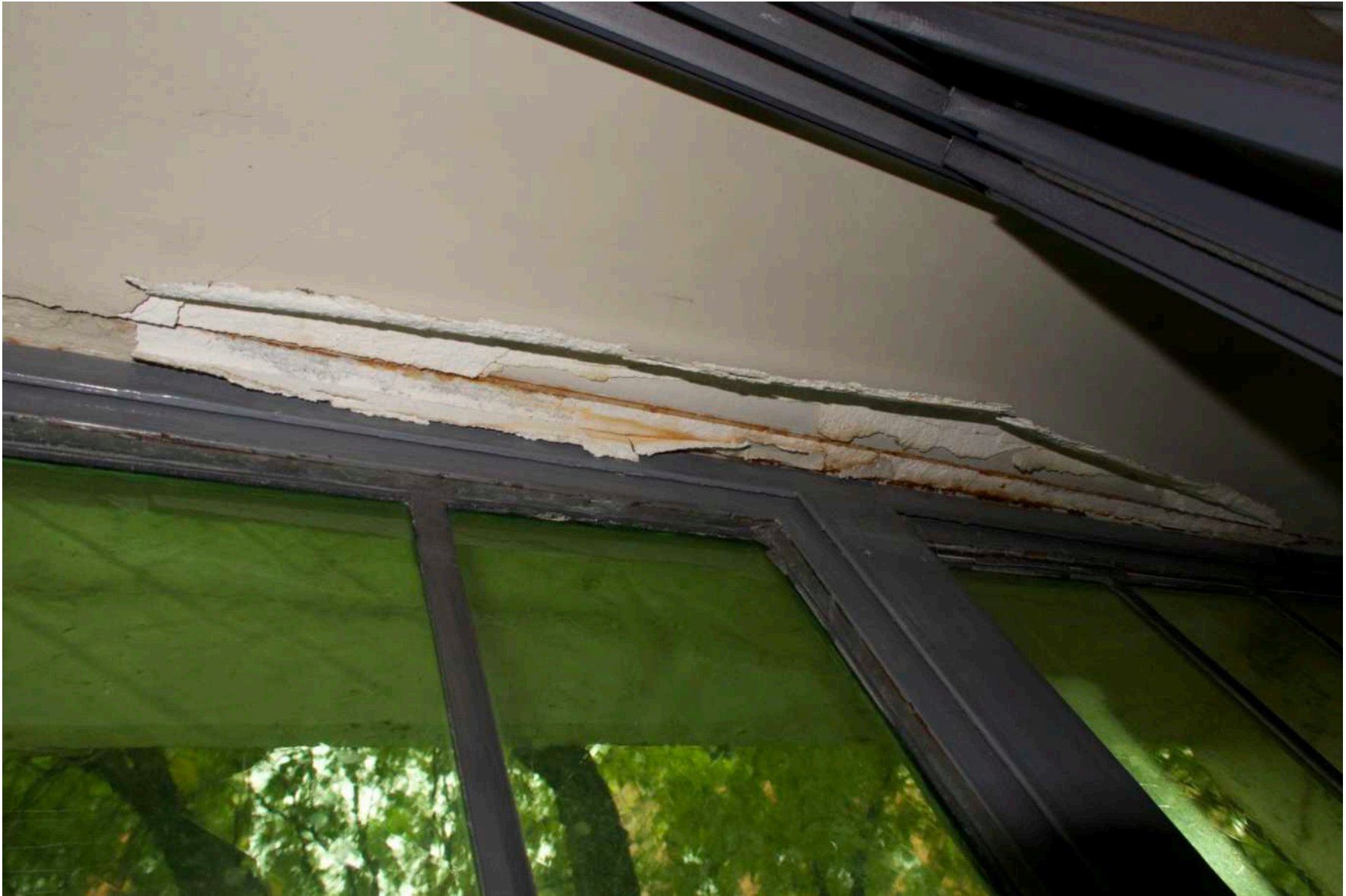
Window 2 and others, universal plaster damages.
