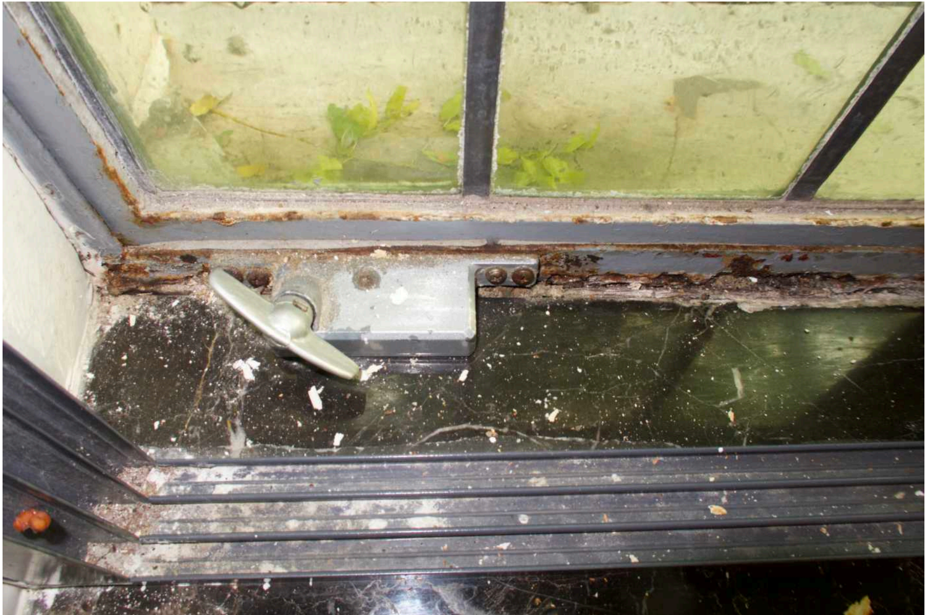
Window 4, hinges and frames rusting.
