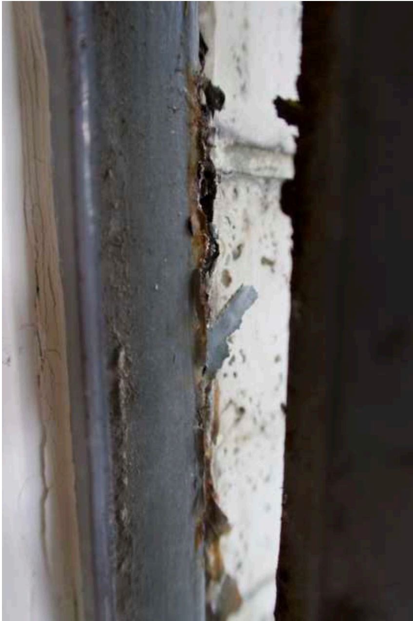
Window 5, frames rusting.
