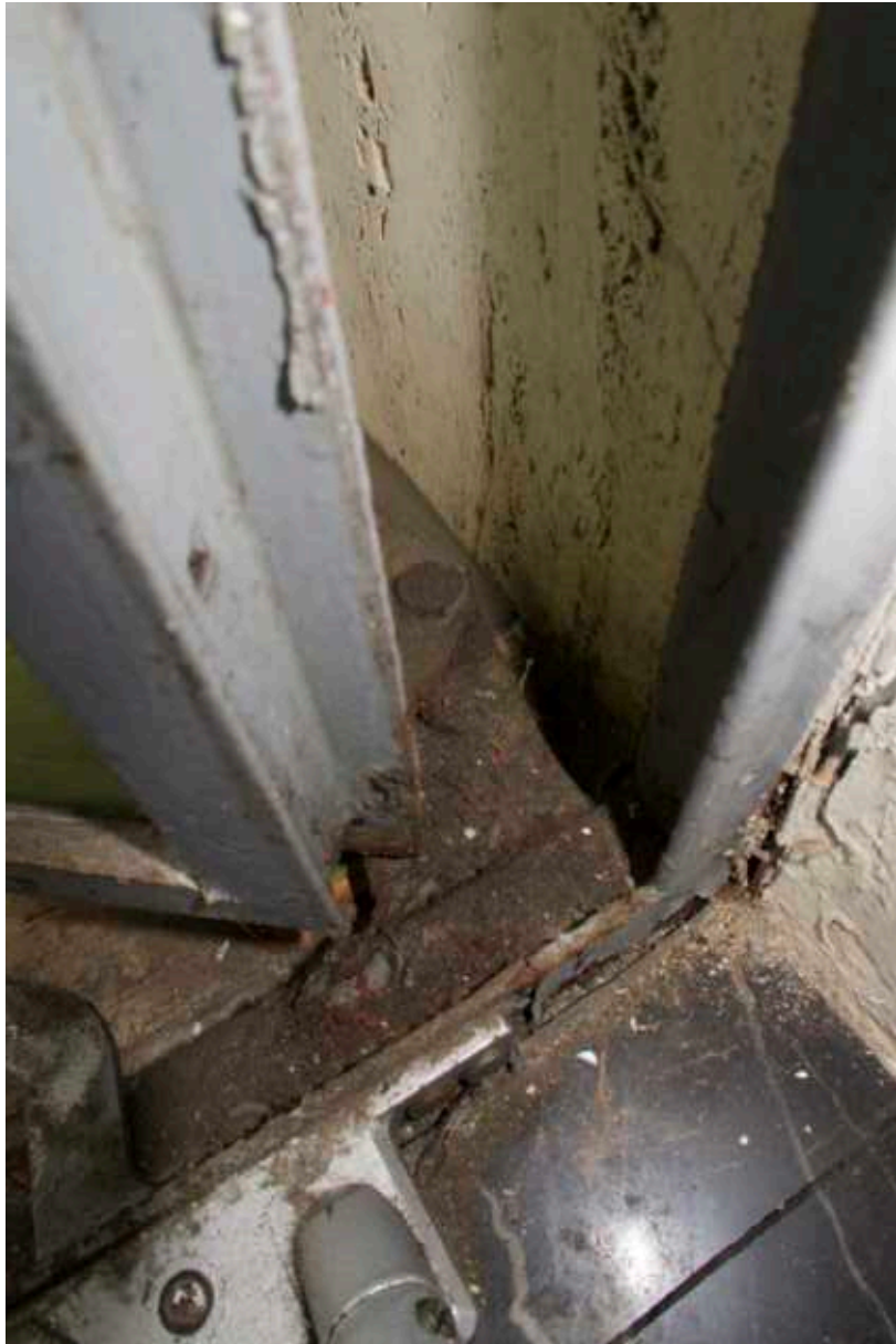
Window 2, hinges and frame rust
