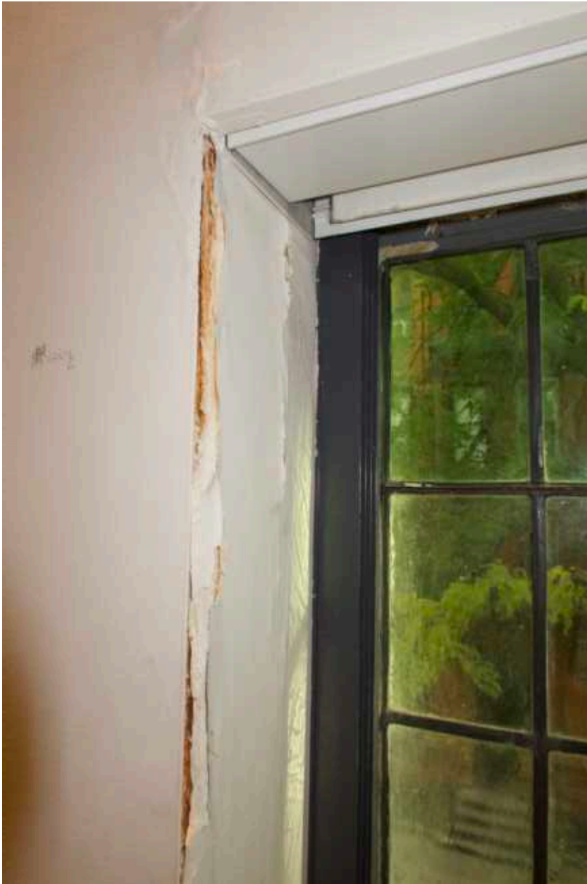
Window 4, plaster damages
