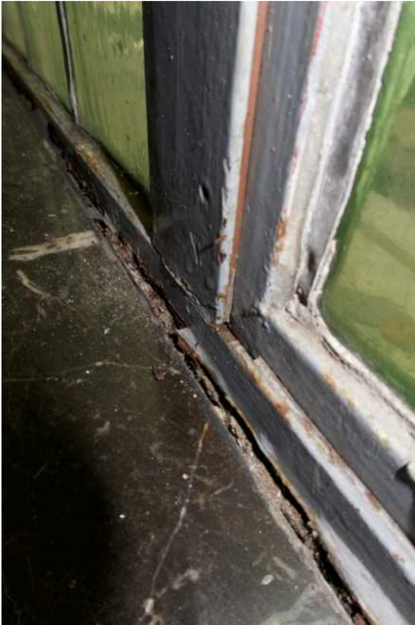
Window 3, frame rust and damage.
