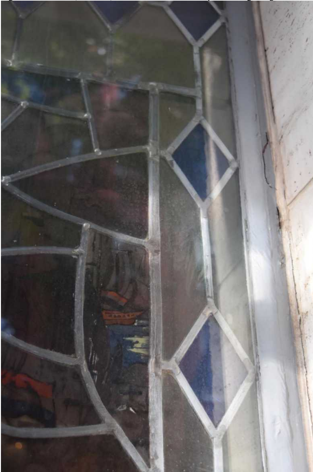
Figure 5: Window 1, Exterior, detail lead corrosion and protective glazing.
