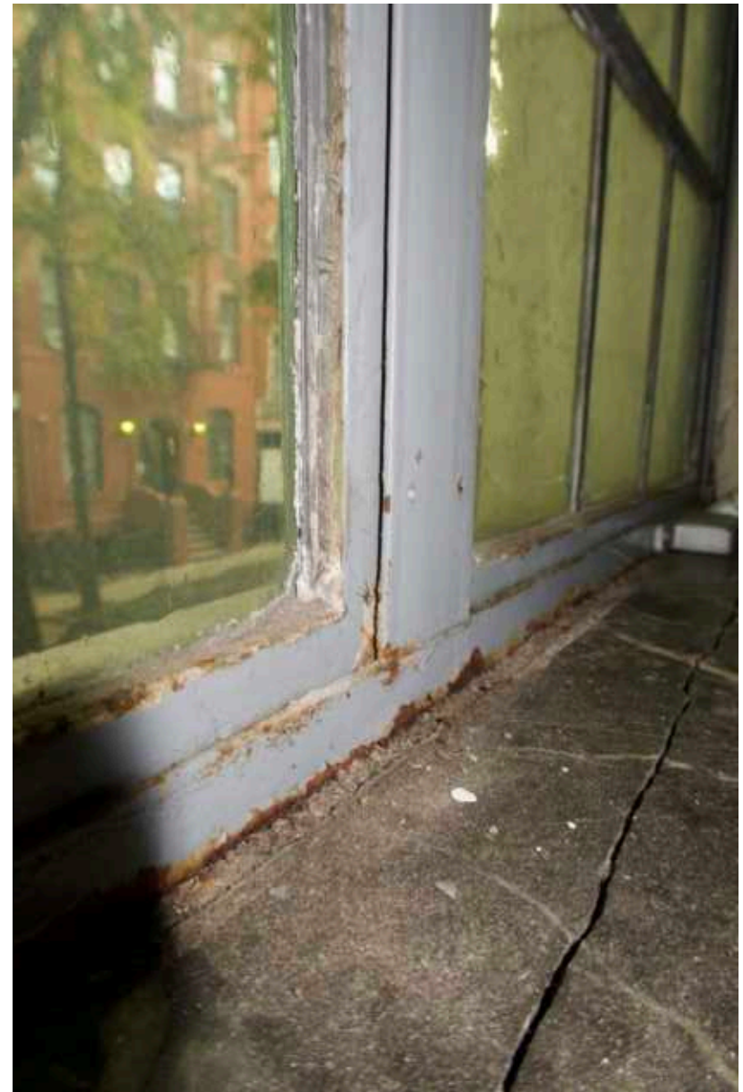
Window 2, frames rusting, marble damage
