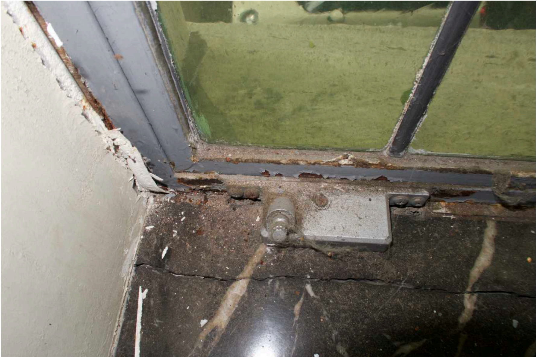
Window 2 and others, universal frames and hinges damages.
