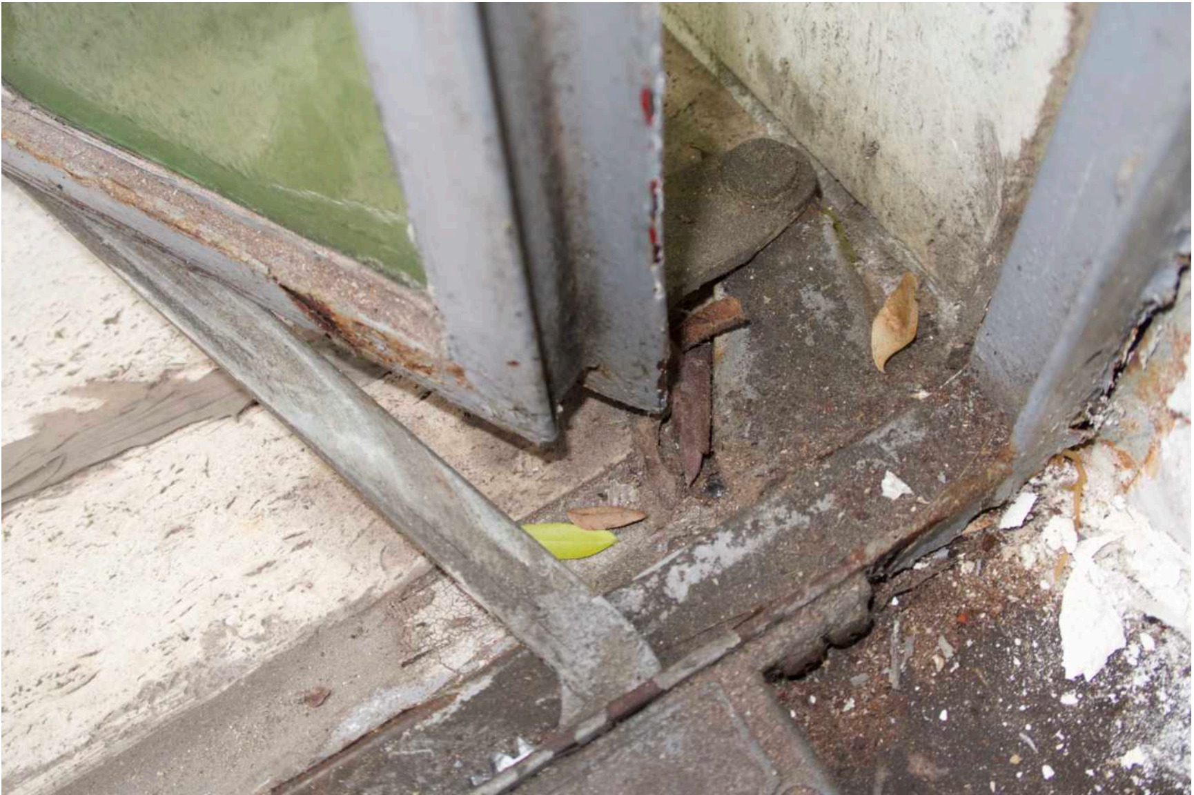
Window 3 and others, frames and hinges damages.
