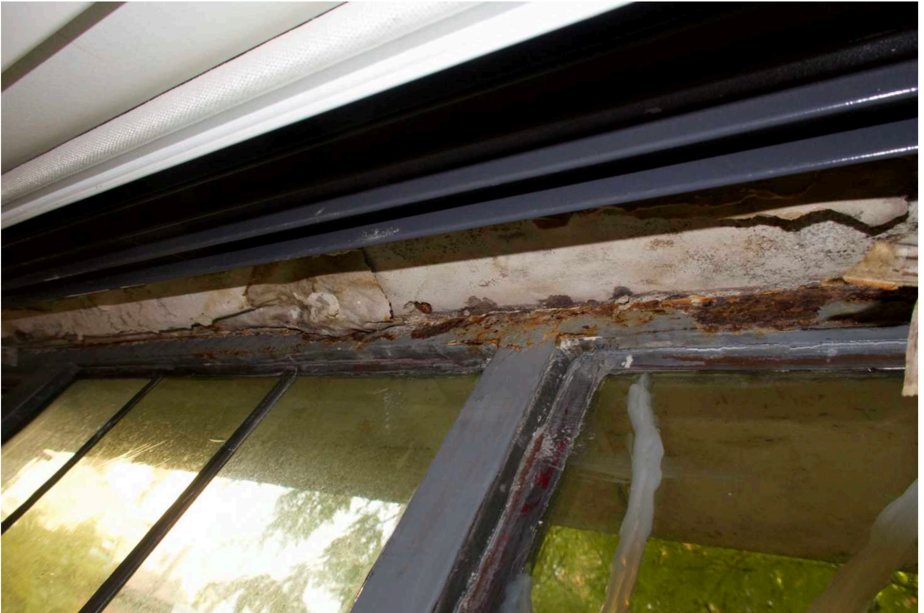
Window 5, broken glass and top plaster damage.
