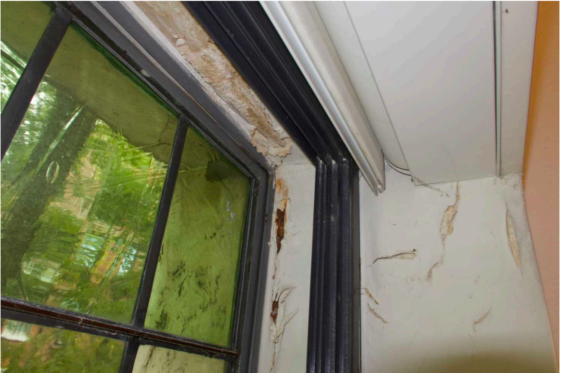
Window 4, severe top and sides plaster damage.
