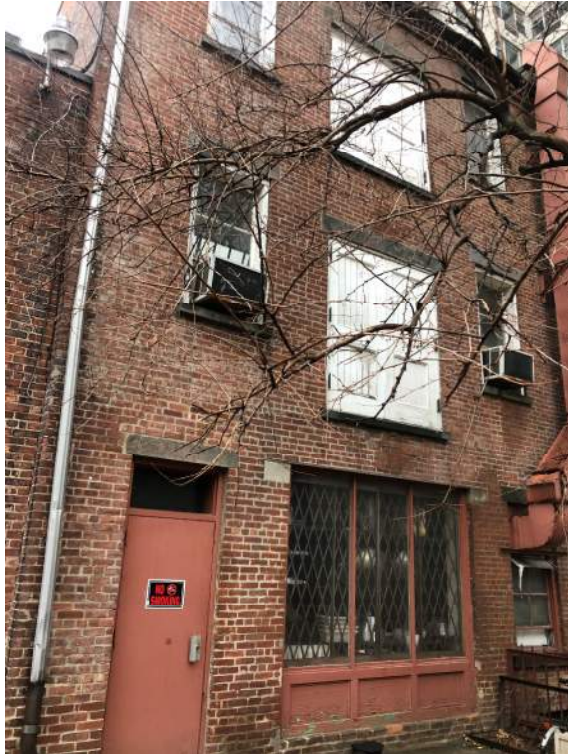
8 West 8 th Street Building elevation north across MacDougal Alley from and facing 19 Washington Square North Rear
