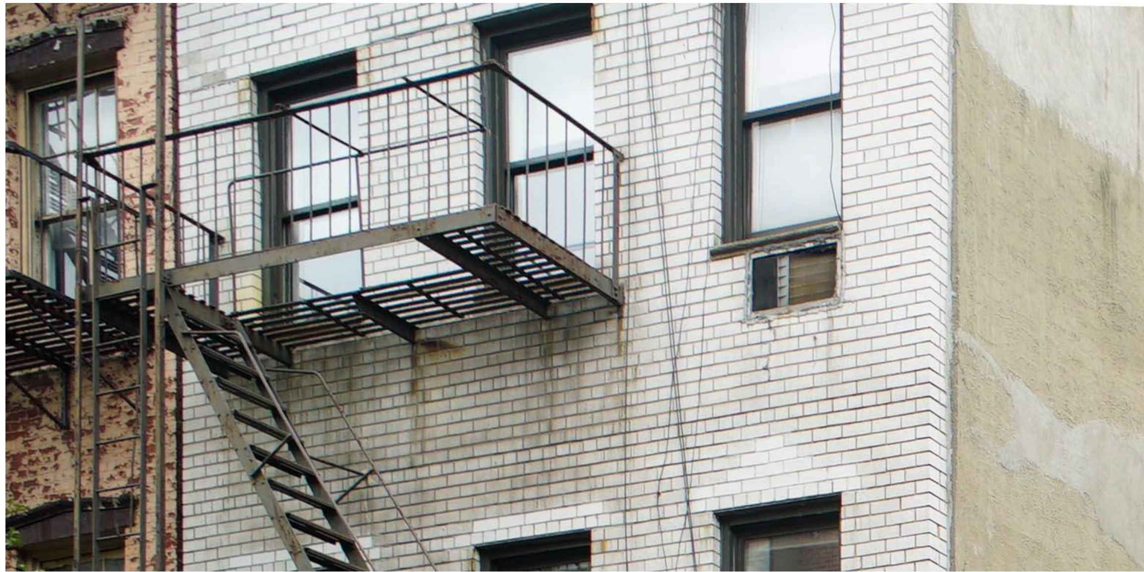
1 - DAMAGED/ CRACKED BRICK IS SEEN ON THE EXTERIOR WALL. RENDERED CEMENT HAS BEEN APPLIED TO SIDE WALL
