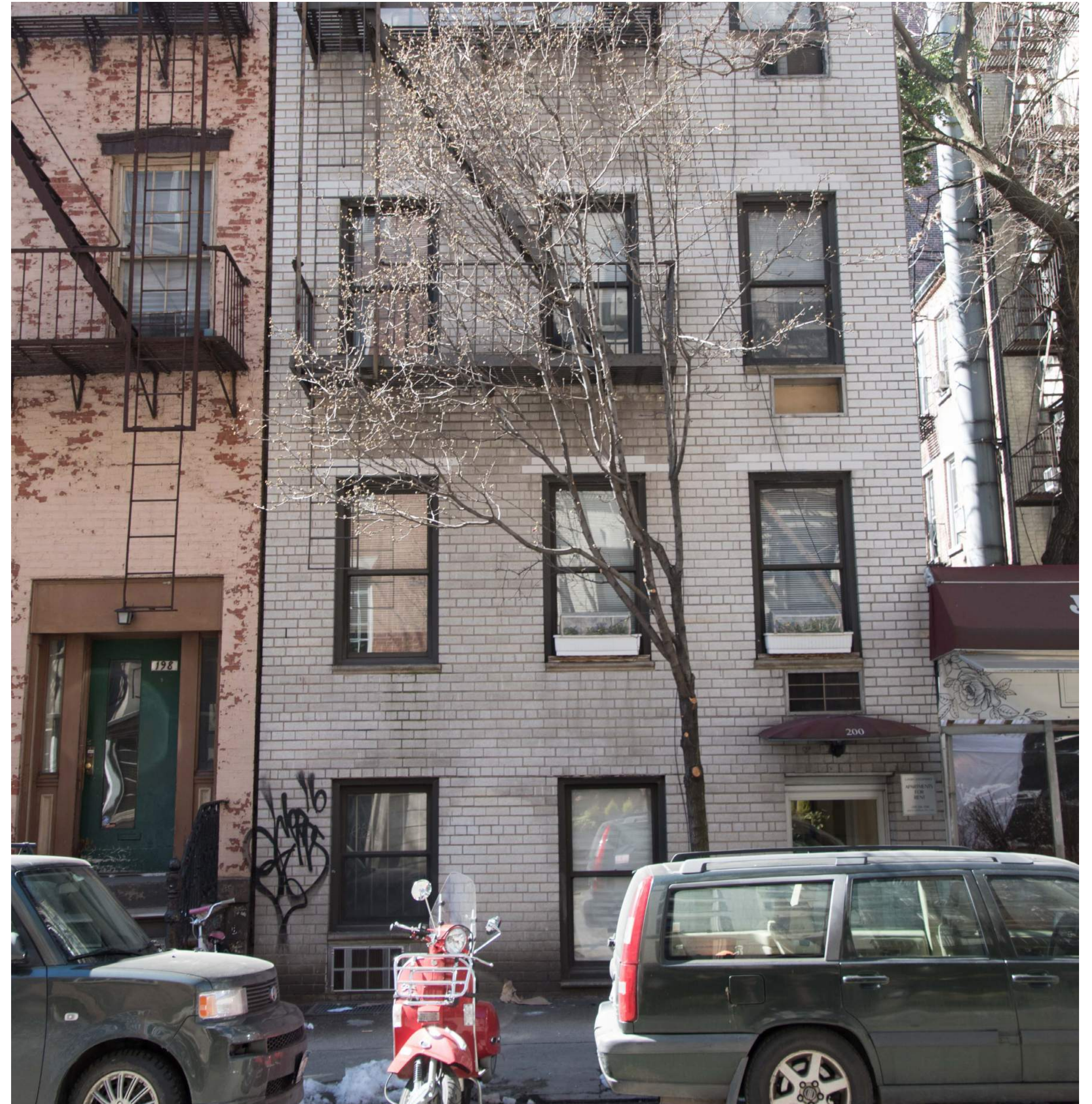
3- AC WINDOW UNITS HAVE BEEN RANDOMLY INTRODUCED INTO THE BRICK WALL
