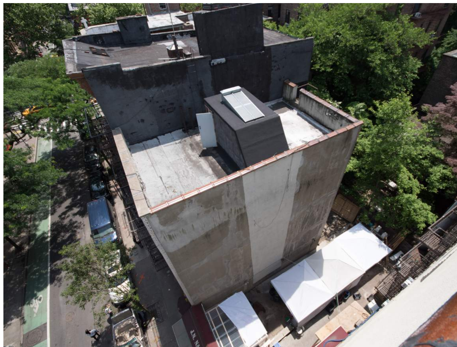
2- VIEW OF 200 PRINCE AND RESPECTIVE YARDS, FROM ROOF OF 202 AVE. OF THE AMERICAS
