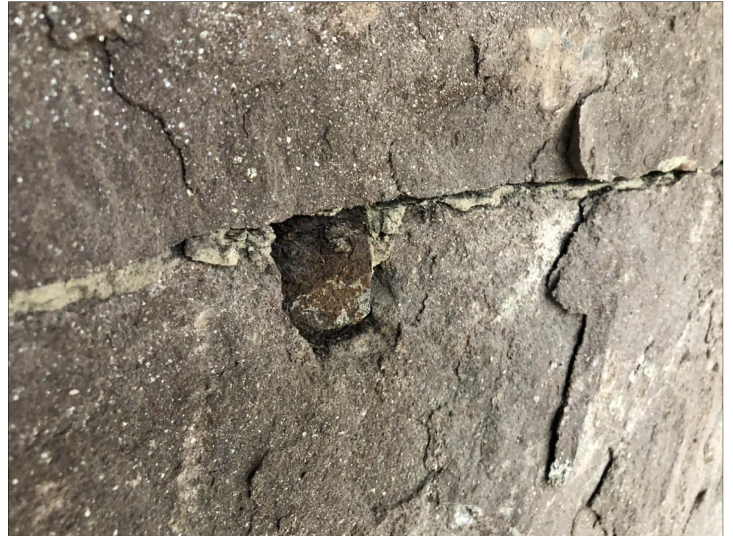
CORRODED VENEER TIE W/ SPALLED BROWNSTONE AT NO. 36
