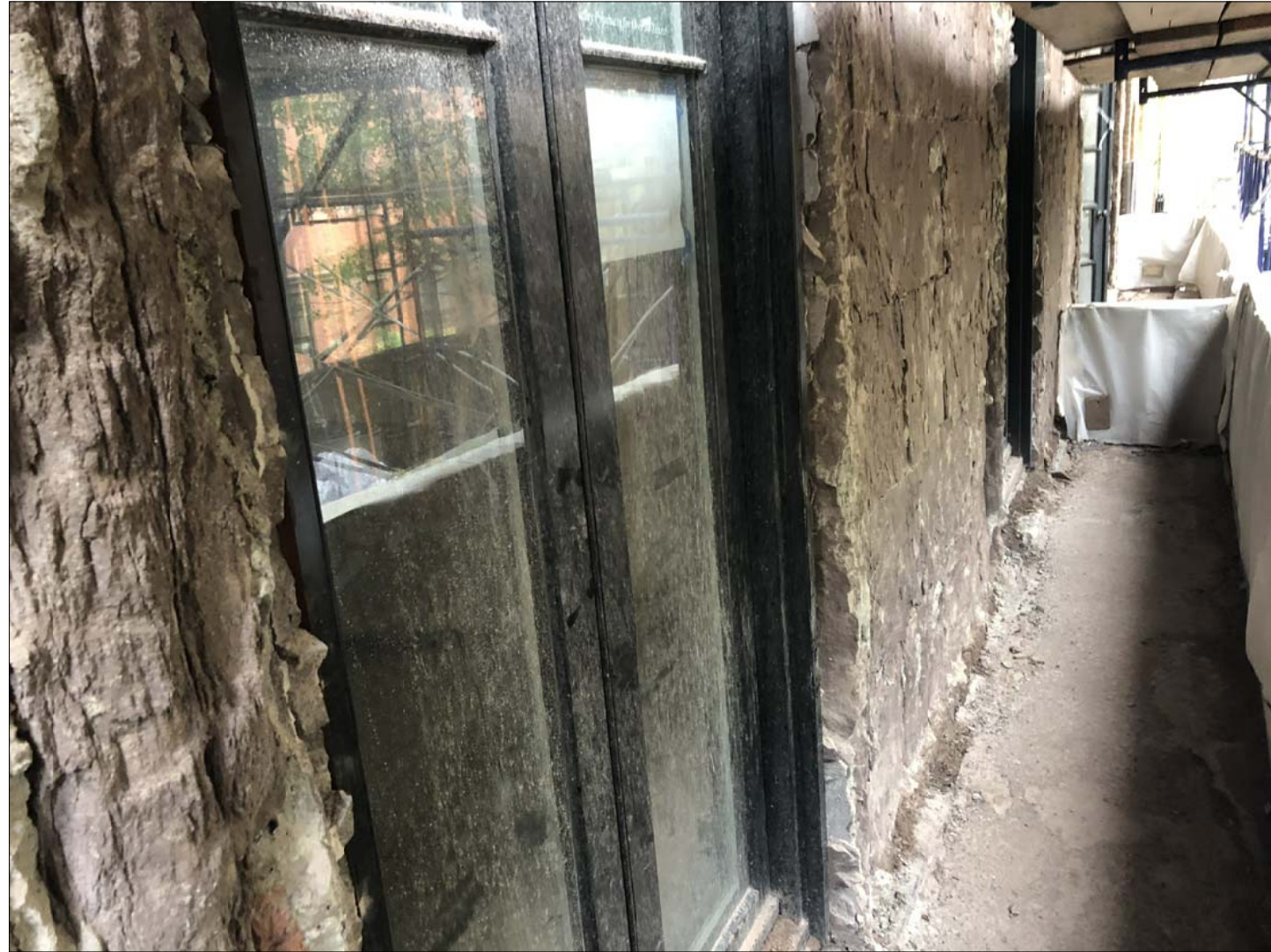
2ND FLOOR EXISTING DETERIORATED BROWNSTONE AT NO. 36
