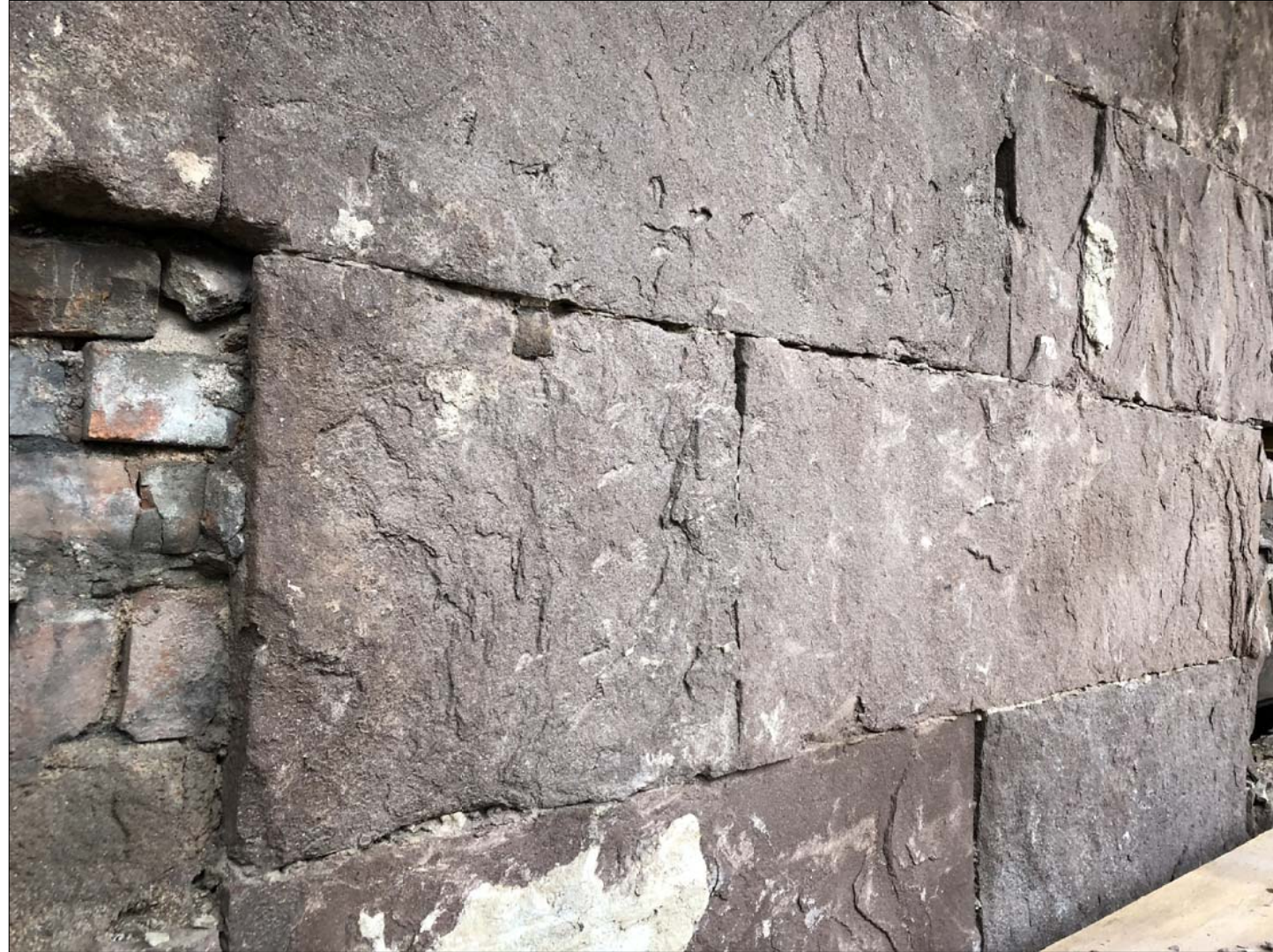
3RD FLOOR EXISTING DETERIORATED BROWNSTONE AT NO. 36
