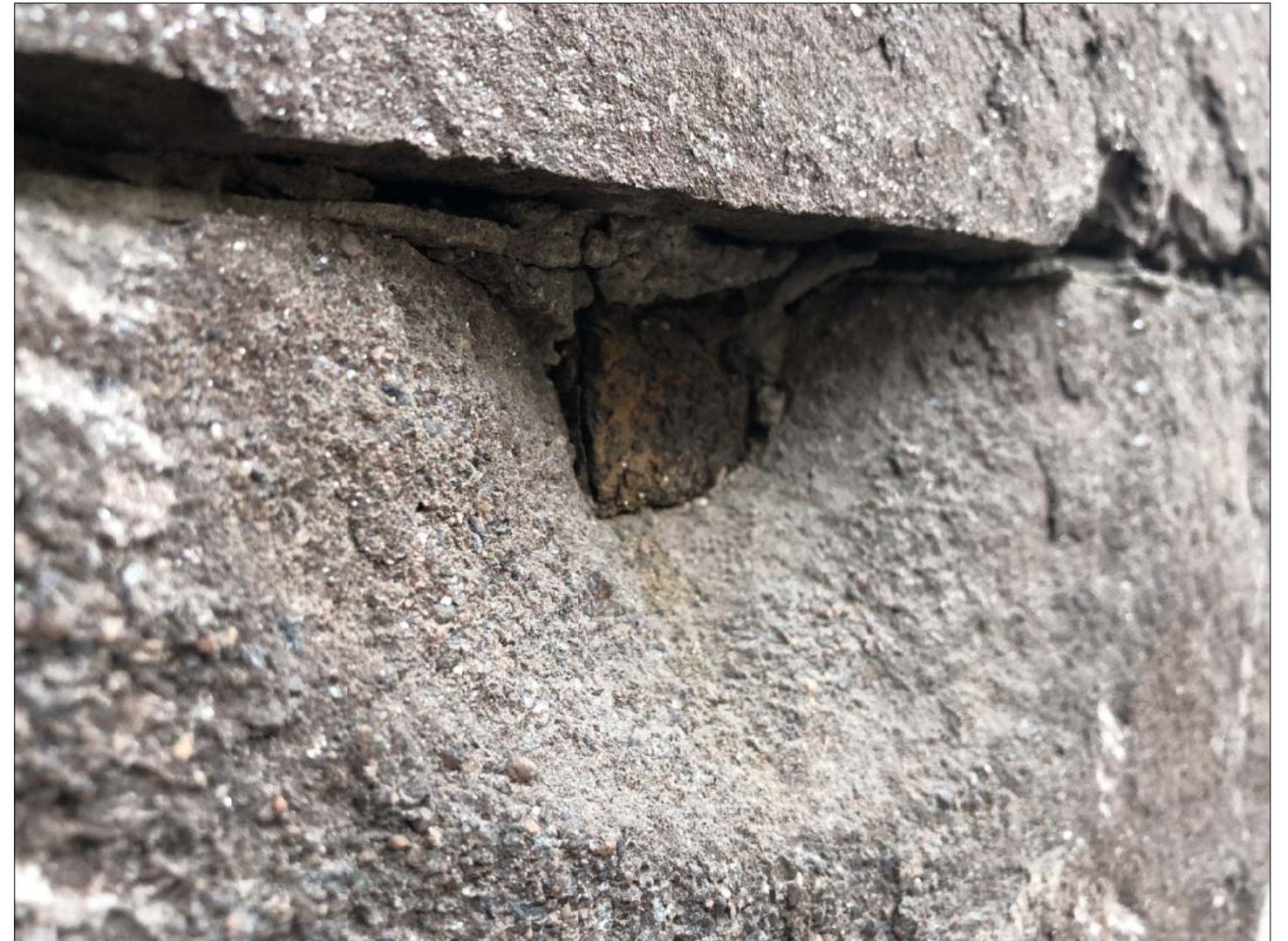
CORRODED VENEER TIE W/ SPALLED BROWNSTONE AT NO. 38
