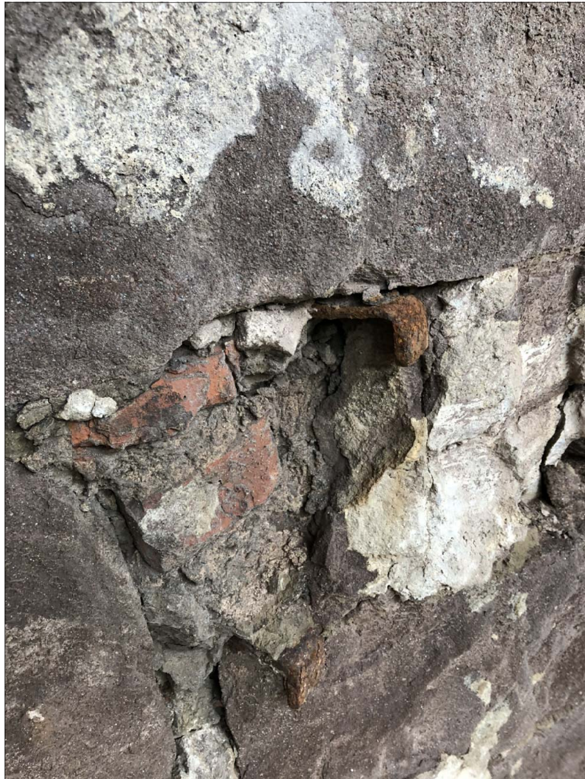
CORRODED VENEER TIE AT NO. 38
