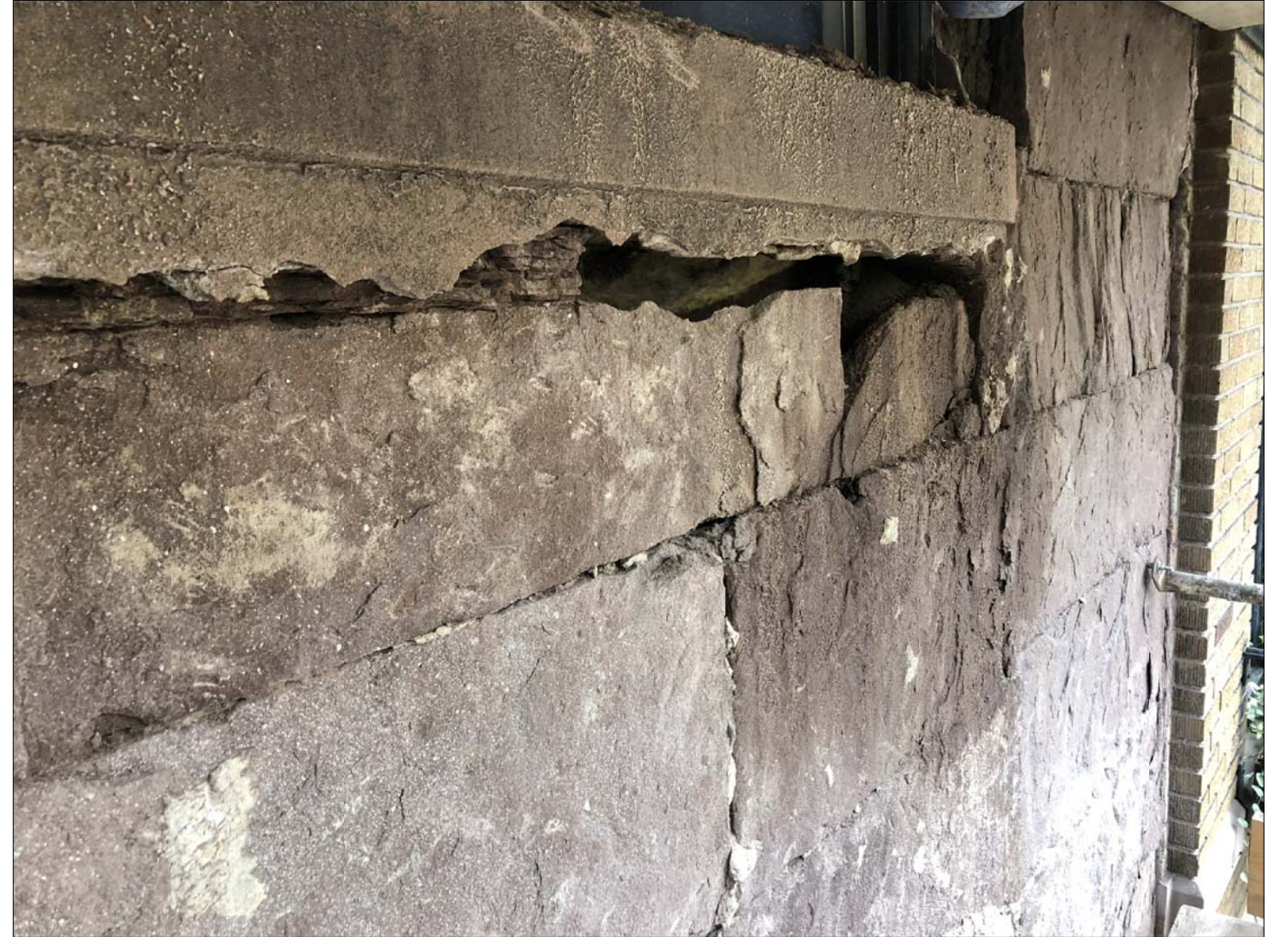
3RD FLOOR EXISTING DETERIORATED / HOLLOW BROWNSTONE AT NO. 38
