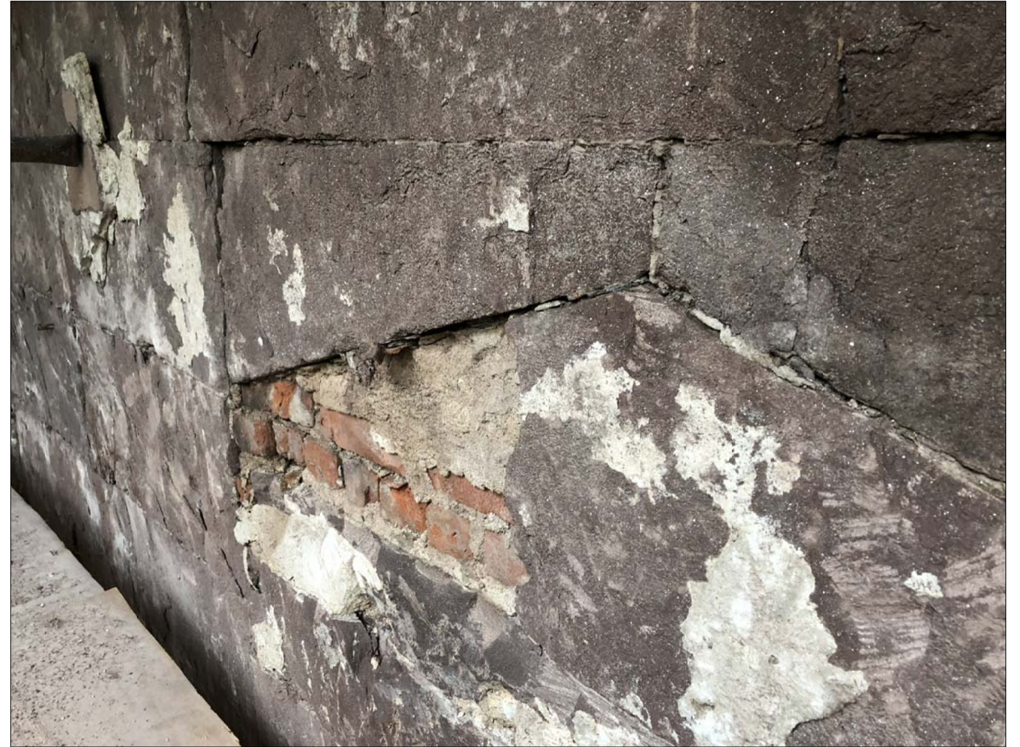
2ND FLOOR EXISTING DETERIORATED BROWNSTONE AT NO. 38
