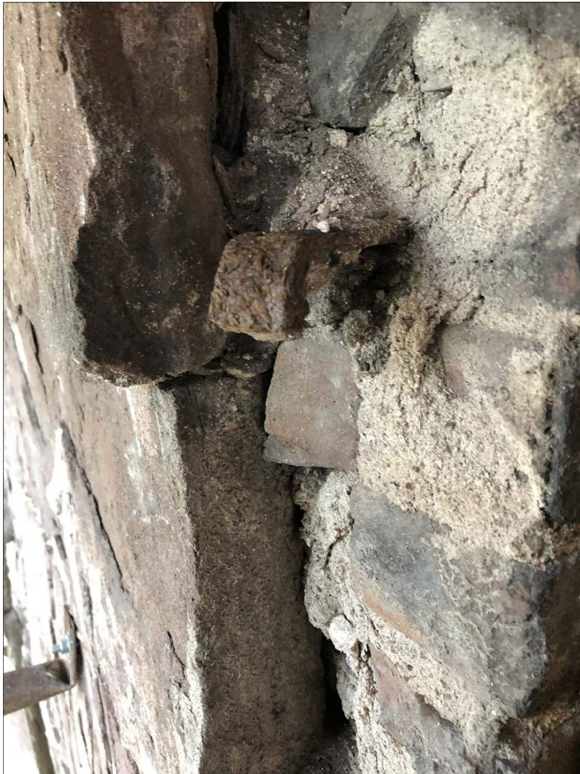
CORRODED VENEER TIE AT NO. 36
