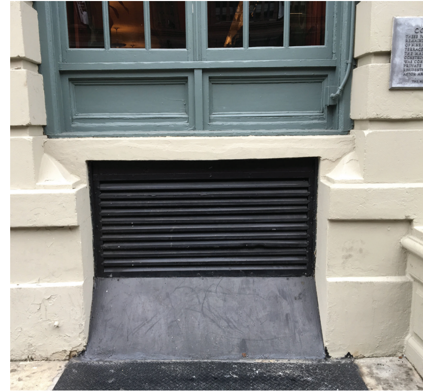
430 Lafayette Existing HVAC
