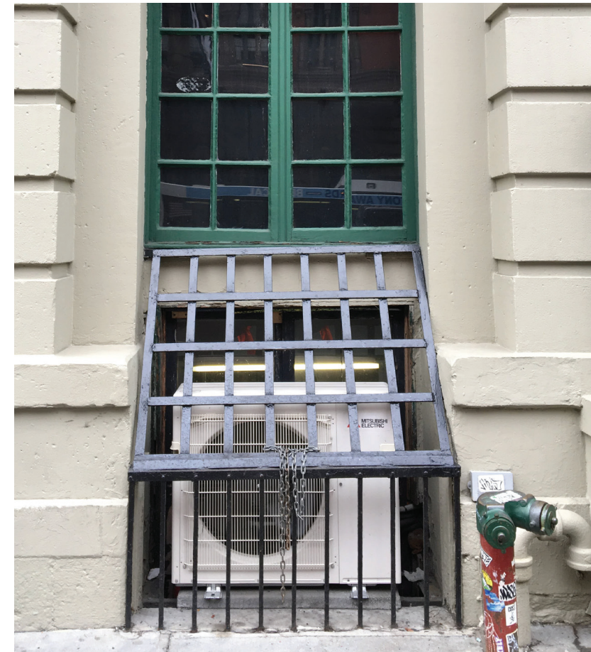
432 Lafayette Existing HVAC
