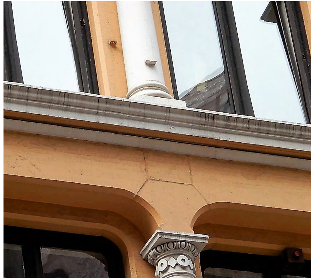
FACADE WITH EXTRANEIOUS HARDWARE, OPEN JOINTS, FLAKING PAINT
