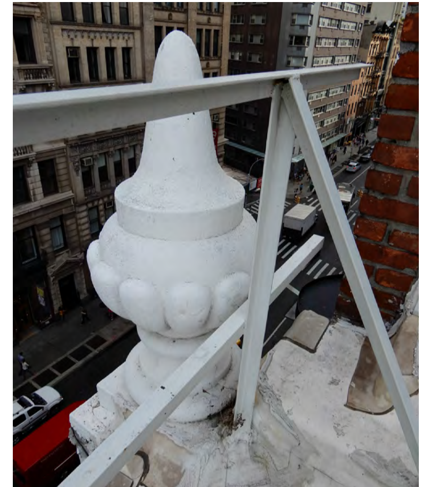
STONE FINIAL AT ROOF HEAVILY COATED, RAIL PIERCING BASE
