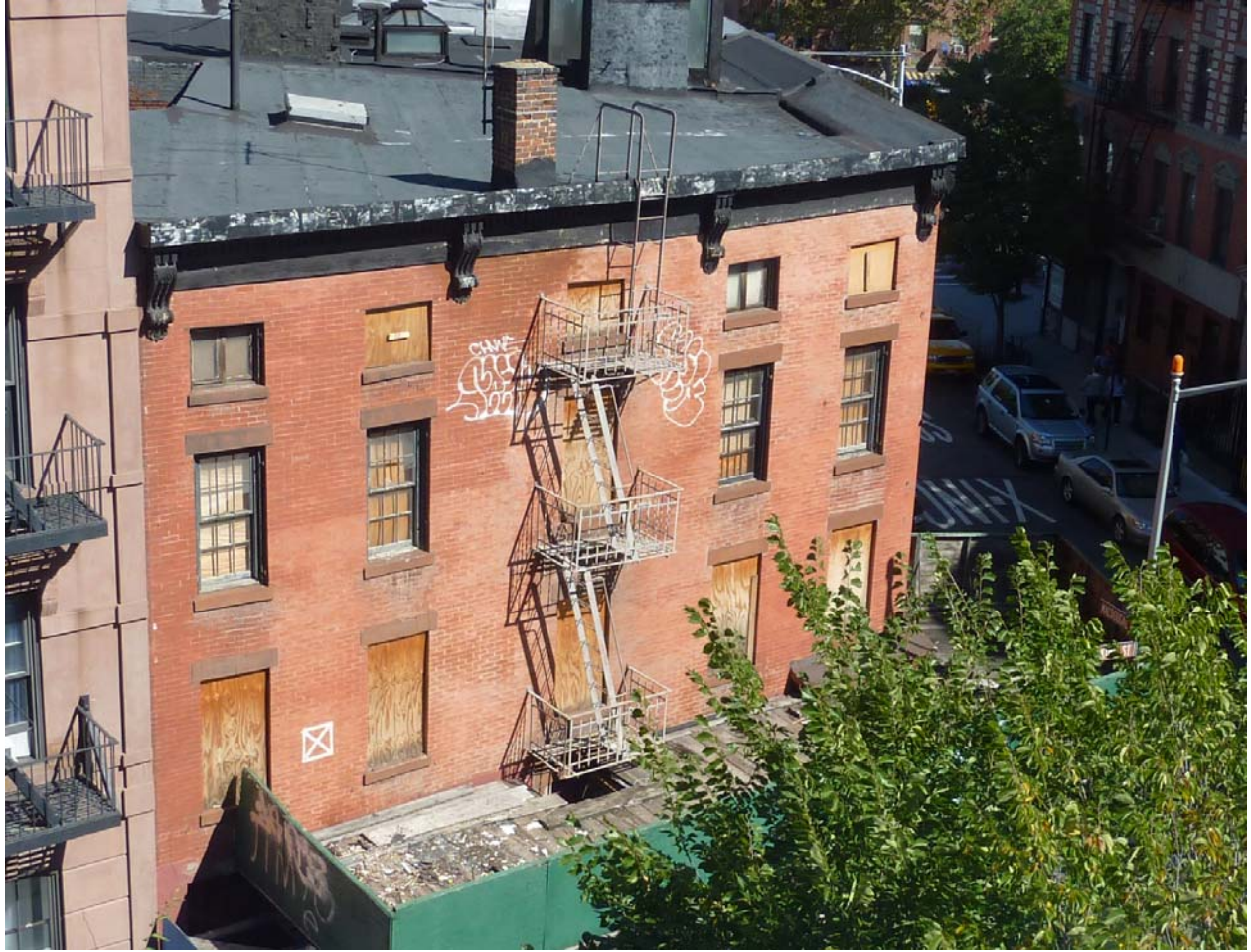
October 2010: Graffiti and water stains remain, upper-right window missing
