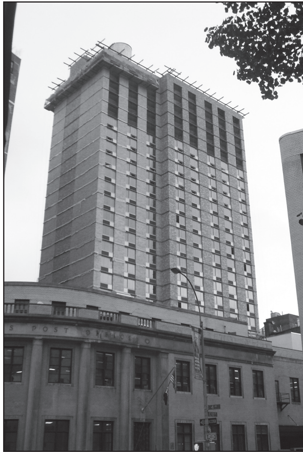
NYU's 26-story mega-dorm under construction on East 12th Street. The university's projected growth over the next 25 years is the equivalent of thirty-four more of these.
